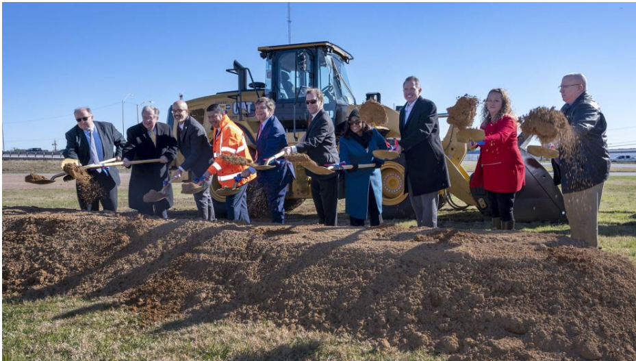
Local officials recently participated in a groundbreaking ceremony to mark the beginning of the Southeast Connector project in Fort Worth.
