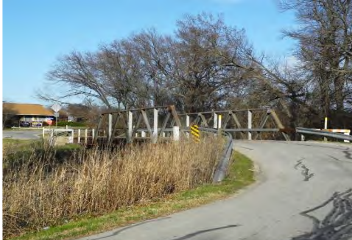
Character of existing bridge over Waxahachie Creek on Zion Road in Midlothian.
