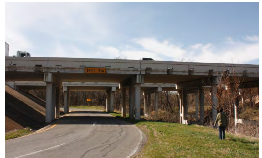
Opportunity for trail to pass under existing I-35E frontage next to Waxahachie creek.
