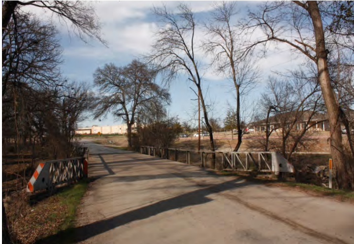
Existing F.M. Road 875 near the north side of the proposed Kemp Ranch development.
