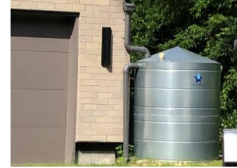
RAINWATER HARVESTING CISTERN
