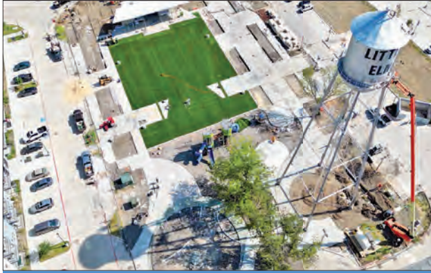
The Lawn at The Lakefront is currently under construction in Little Elm. COURTESY OF THE TOWN OF LITTLE ELM
