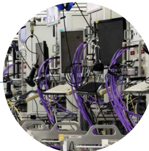
Automated factories and DCs
