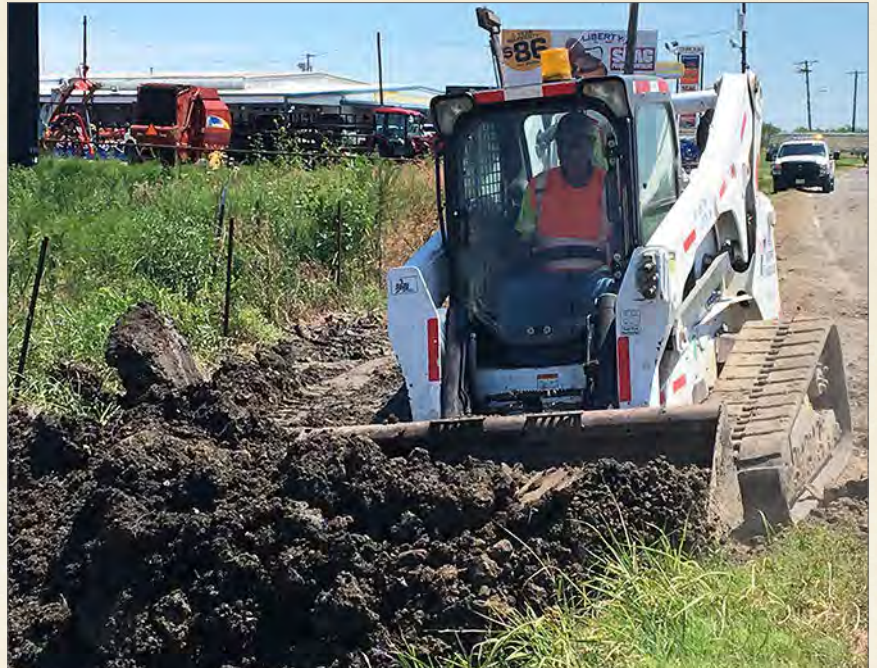
Alan Malone operates a small track-type tractor while doing ditch shoulder work in Royse City.
