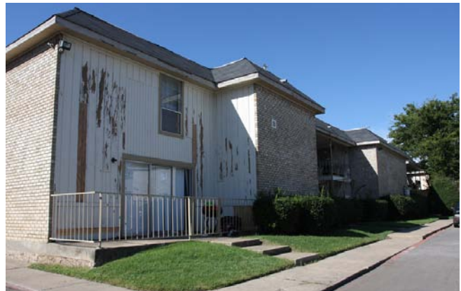
Image 2: Lack of maintenance detracts from the value of residential properties.
