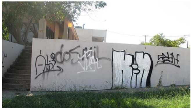
Image 12: Vandalism occurs on private and public property.
