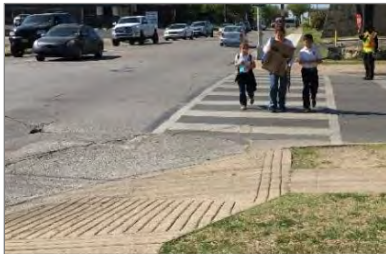
7. Curb Ramp Not Contained in Crosswalk
