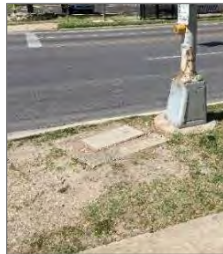
7. Lack of Landing Pad
