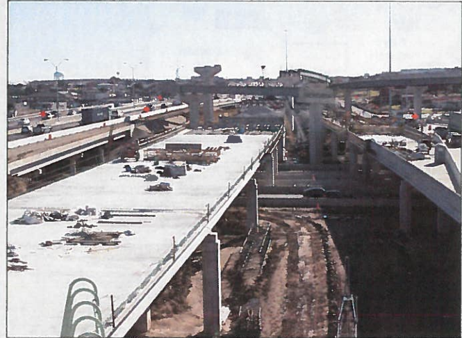
Construction on the I-30/SH 360 Interchange Project in Arlington. The $233 million project will increase safety, connectivity and mobility for motorists.
