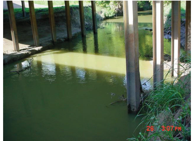
Photo shows the creek under the C. F. Hawn Frwy; facing upstream
