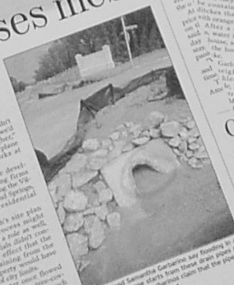
Anthony and Samantha Garbarino lay flooding in and around their home starts from their drain pipes near their property. The Garbarinos claim that the pipes are undersized and not maintained.
