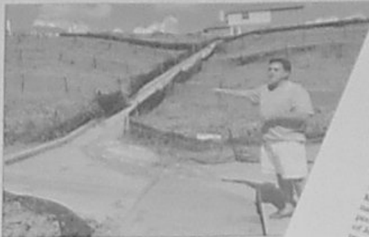
In this July photo, Craig Sullivan points out concrete frames along the hillside. The Dallas runoff water from a new neighborhood into a storm drain Sullivan says runoff water has destabilized his home's foundation.
