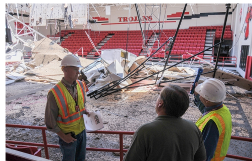
Preliminary damage assessment at West High School (FEMA)
