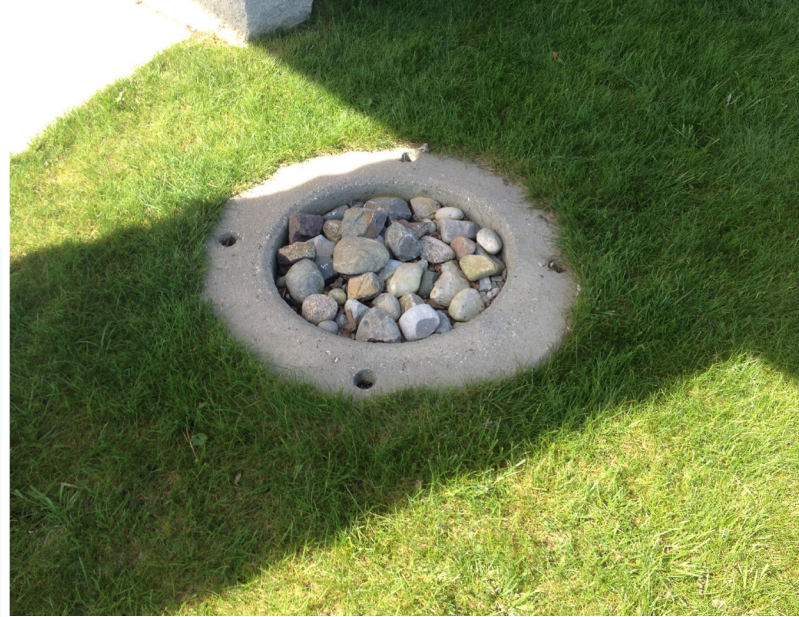
Downspout Drywell in Traverse City, MI. (Source: Tetra Tech)
