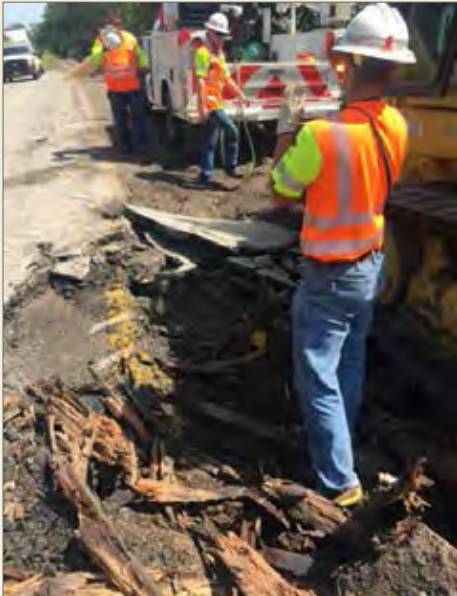
Javier Trevino, Philip Newby and Nathan Fojt were doing base repair on FM 1389, when they discovered the remains of an old railroad.
