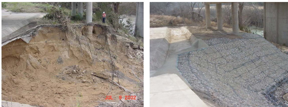
Figure 26. FM 474 @ Guadalupe River in the San Antonio District—Erosion Repairs and Installation of Embankment Protection Measures (Gabion Mattresses).
