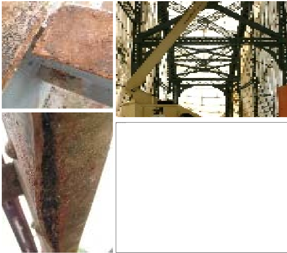
Figure 37. Typical Steel Painting Project, Showing Localized Defects (Left), the Bridge during the Painting (Top Right), and the Bridge after Being Reopened (Bottom Right).
