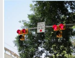
Example of PHBs mounted on a mast arm. Source: FHWA
