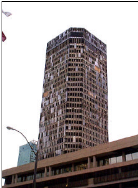
Above: Tornado-damaged Bank One building in downtown Fort Worth. Window replacement alone is expected to cost over 50% of the structure's appraised value.
