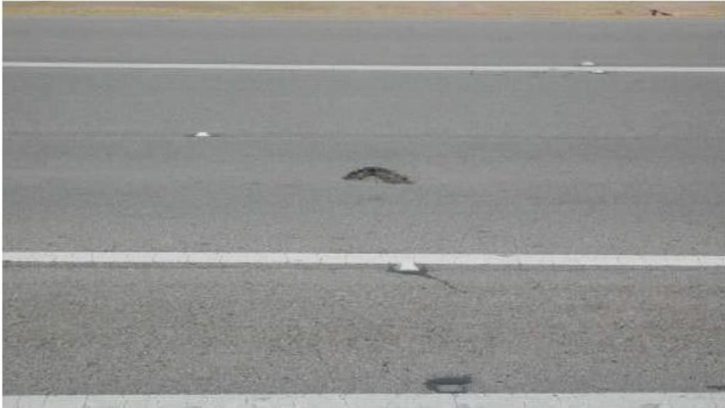
8 - Pothole of 1 sq ft on deck pavement
