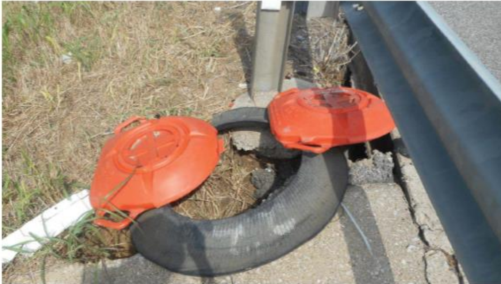
11 - Erosion at Northwest corner embankment
