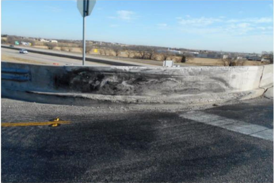
IMPACT DAMAGE ON RECENTLY REPAIRED CONCRETE APPROACH RAIL AT NW CORNER LOOKING NORTHEAST
