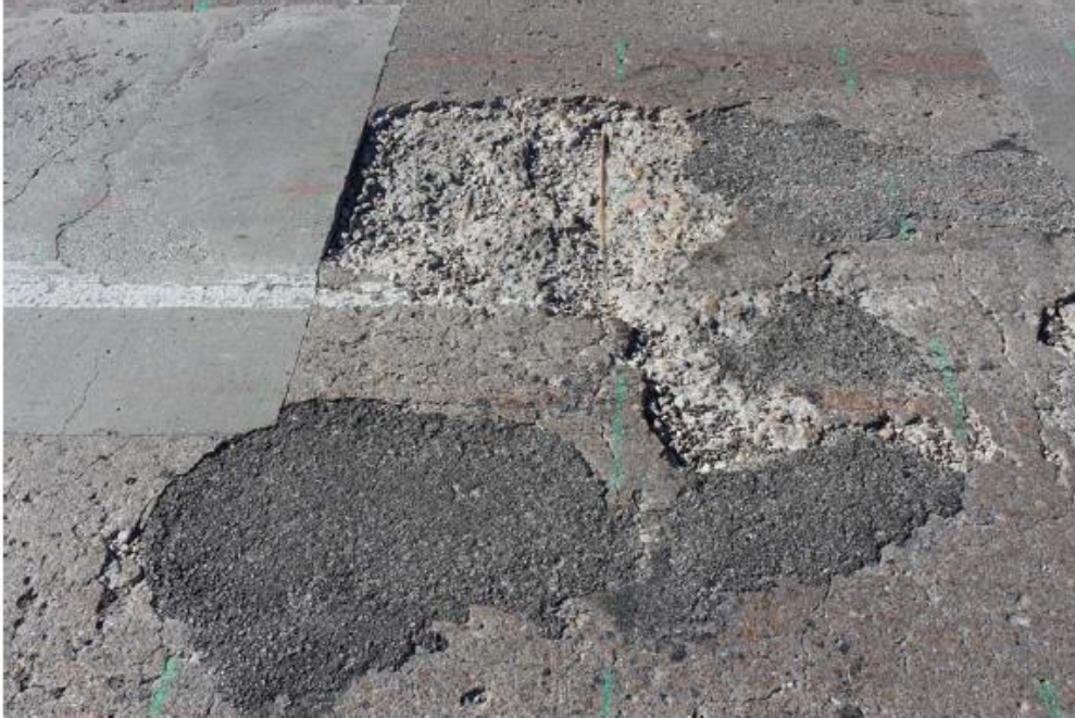
DECK SPALLING SPAN 2
