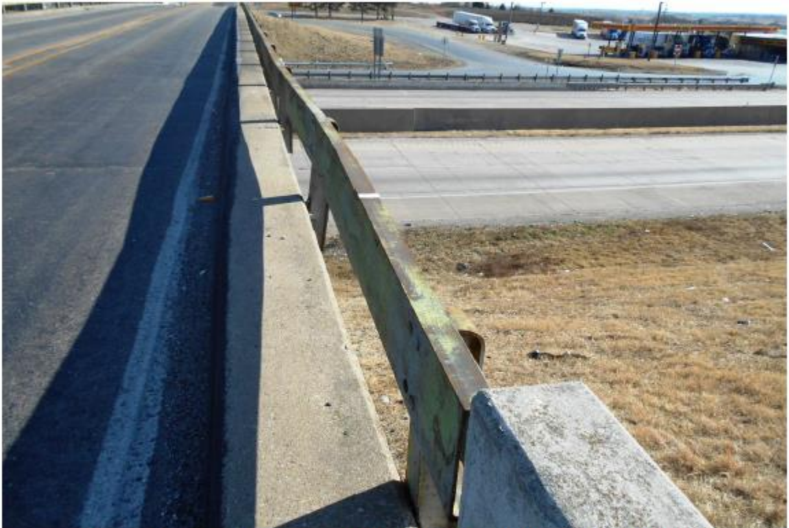
IMPACT DAMAGE TO THE SOUTH BRIDGE RAIL IN SPAN 5 LOOKING EAST
