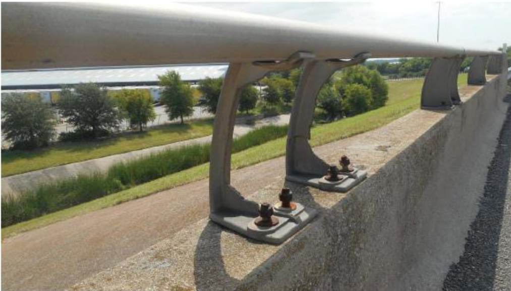
10 - Handrail post damaged in two locations on east bridge rail
