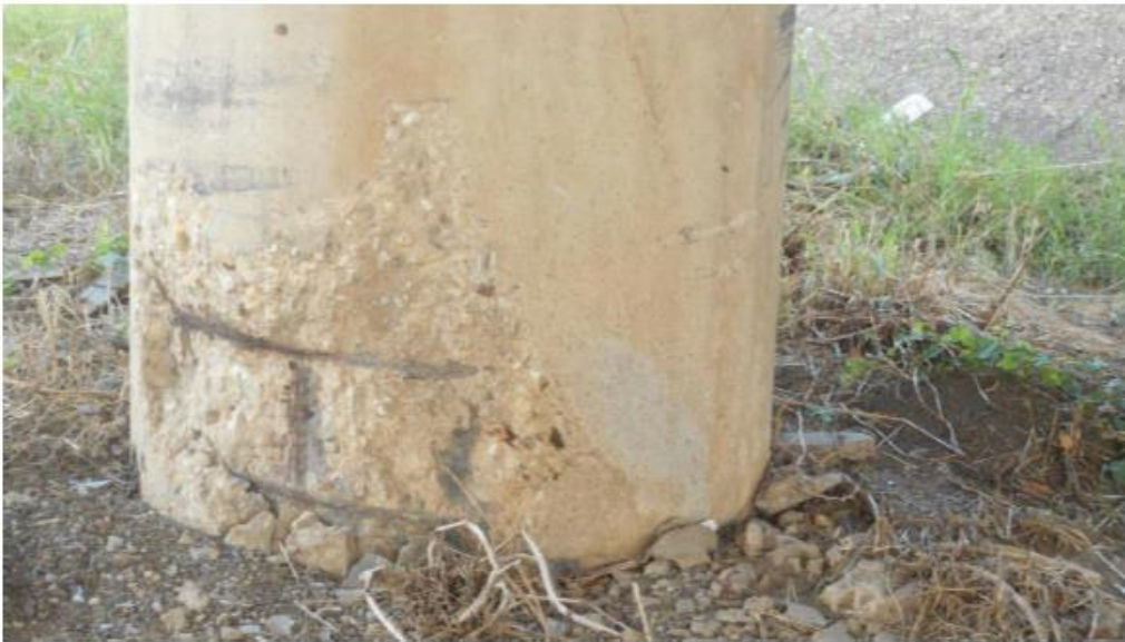
5 - Spall at base of west exterior column in bent 2
