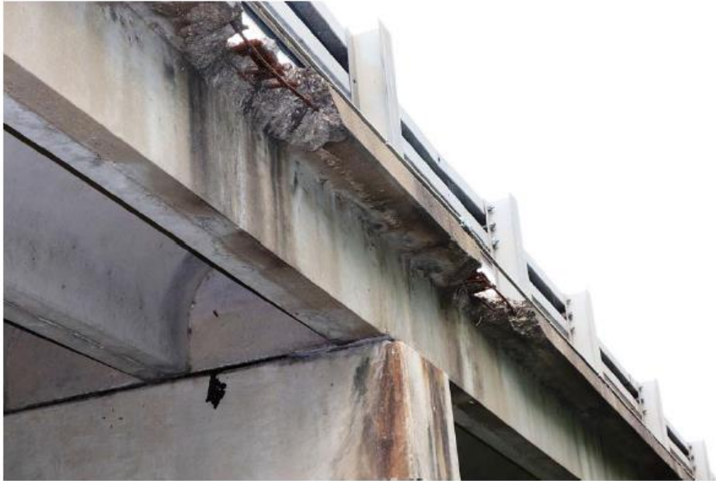
DECK SPALLS Spans 34 & 35
