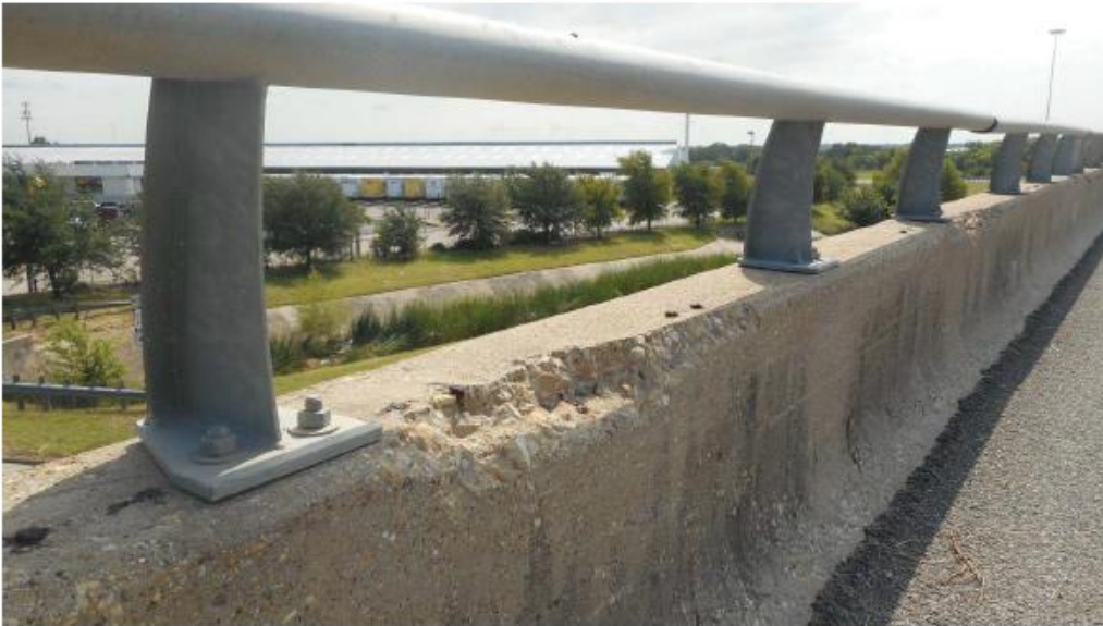
8 - Spall in east concrete bridge rail
