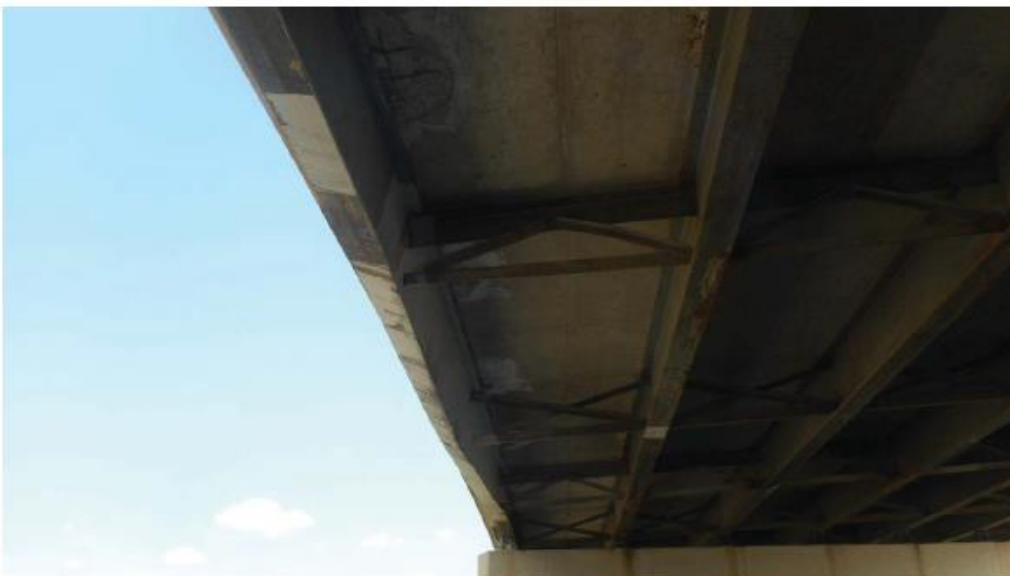
6 - Impact damage to west beams of span 2. Diaphragms hanging. Spalls in deck between beams
