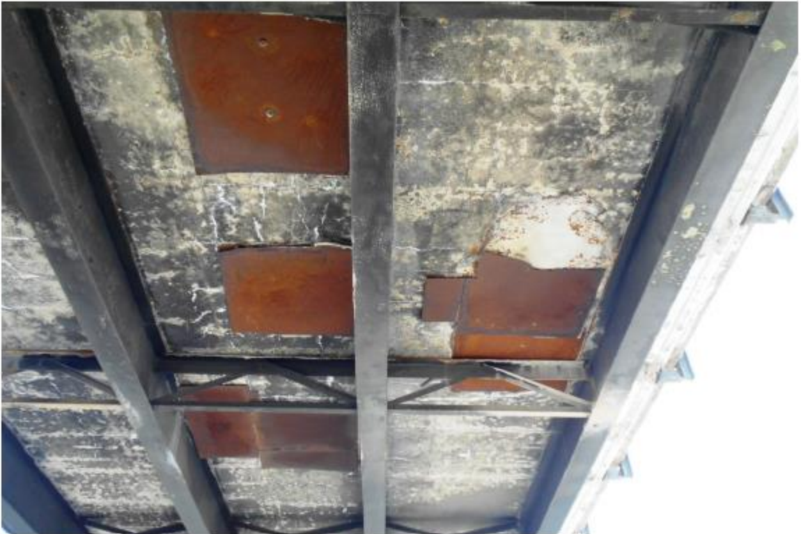
FIRE DAMAGE WITH SMOKE STAINS ON BEAMS AND DECK SOFFIT IN SPAN 4 LOOKING EAST
