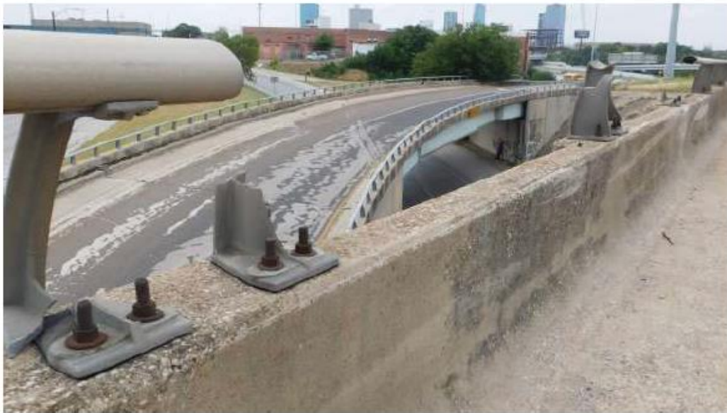
12 - Missing 20 ft tube section on West bridge rail
