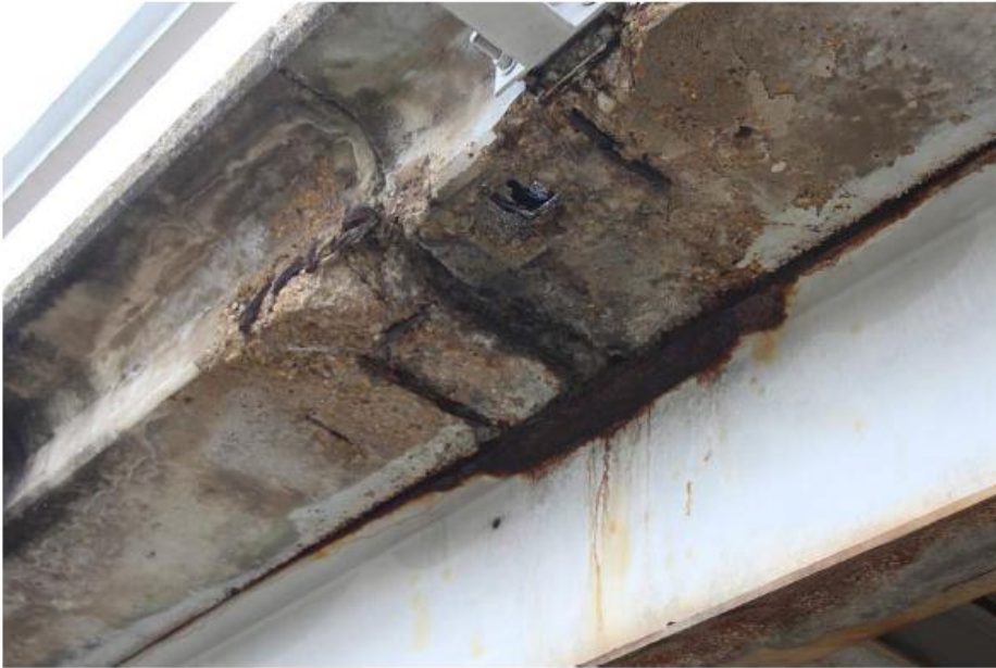
EXPOSED RUSTED REBAR Span 1
