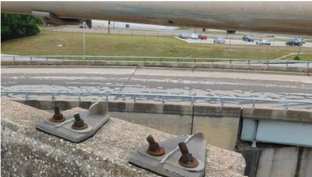
13 - Missing posts on West bridge rail
