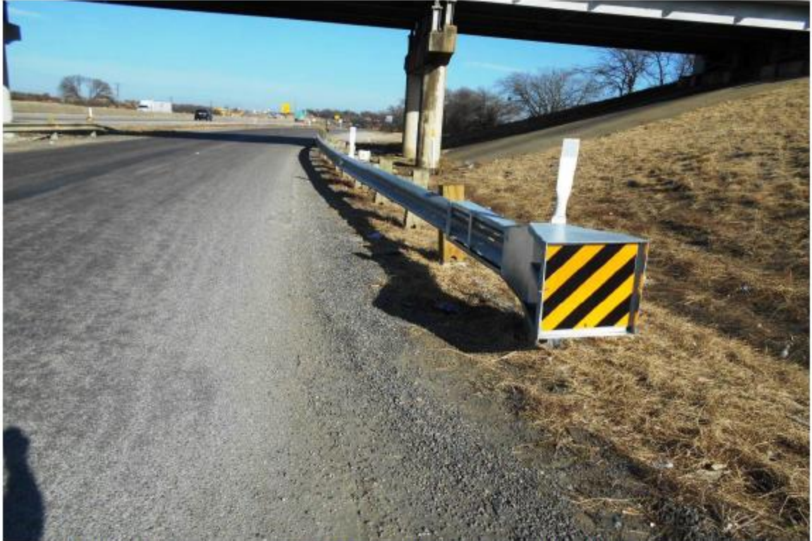
COLLISION PROTECTION SYSTEM OF NBFR AT SE CORNER HAS BEEN REPAIRED LOOKING NORTH
