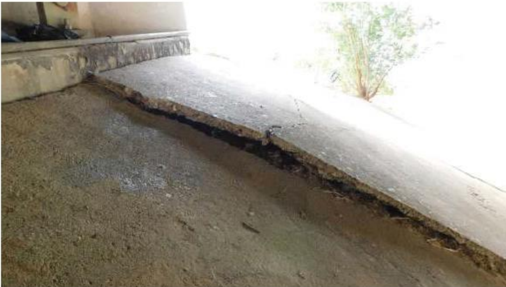
14 - Northeast riprap heaving
