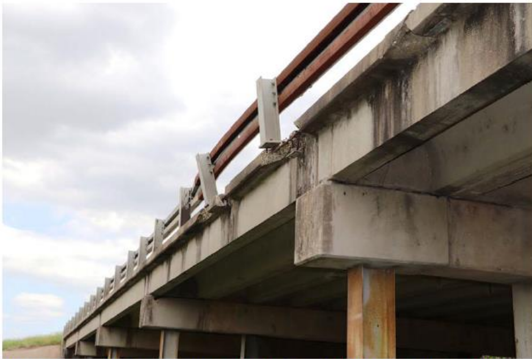
DECK SPALLS Span 43
