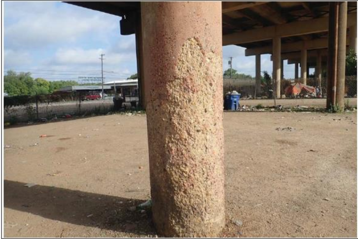
Photo 27 - Bent 15, east column, bottom 6' with 1" D spalling
