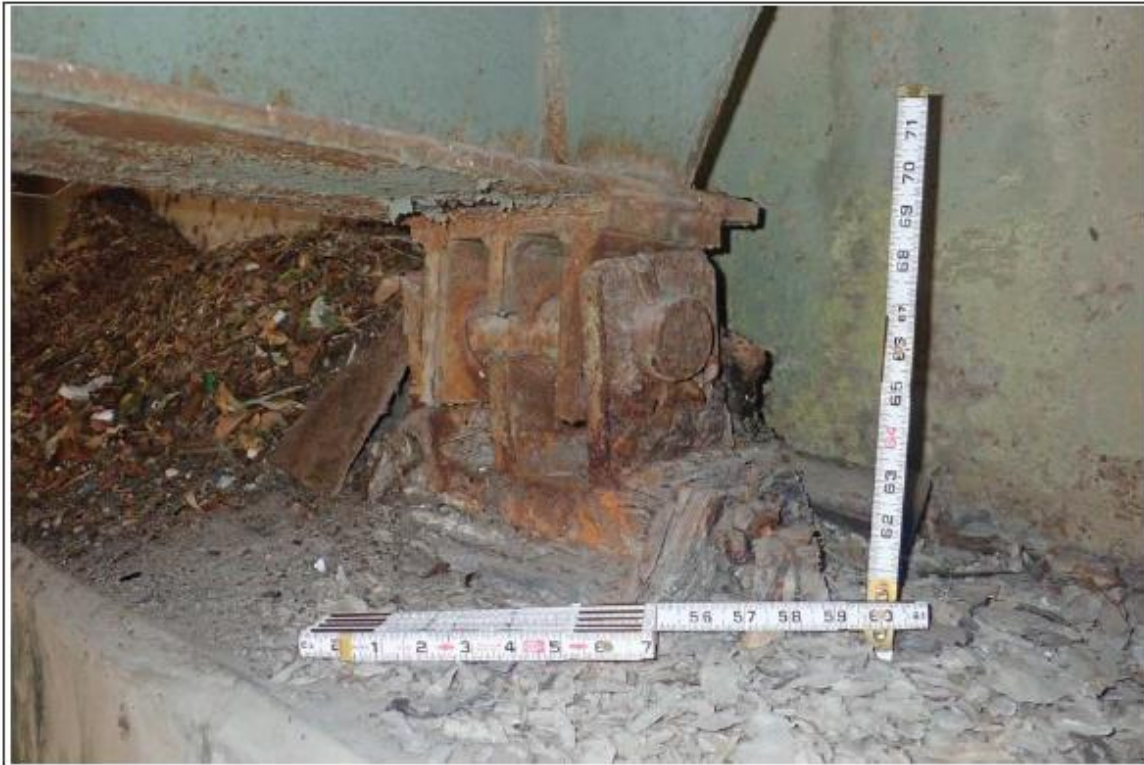
Photo 19 - South abutment, looking east, typical bearing with severe laminar corrosion
