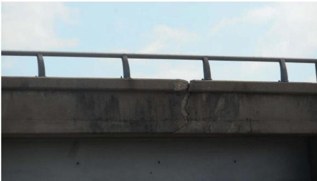
12 - Southwest corner concrete bridge rail has cracks and a spall
