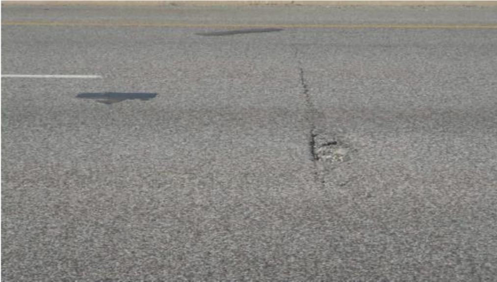
9 - Pothole in deck at span 2
