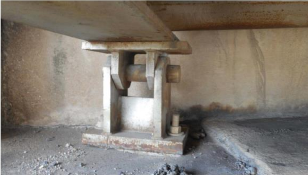
7 - Missing cotter pins at Northwest abutment
