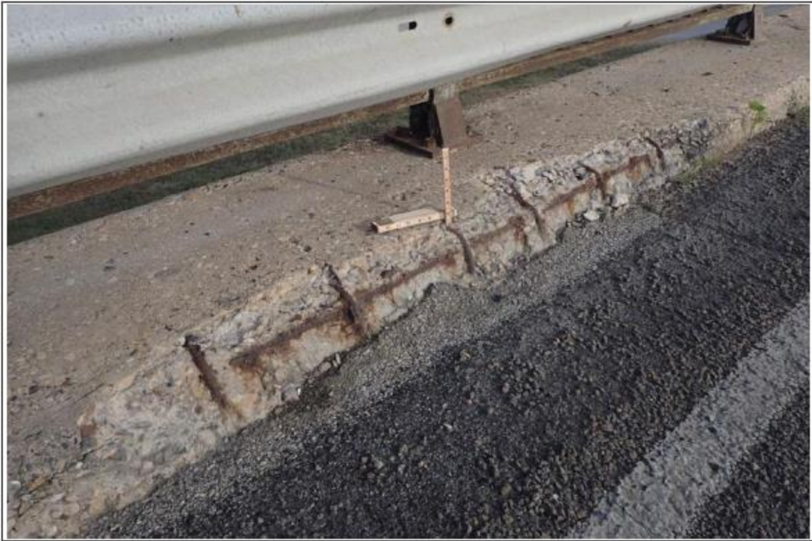
Photo 10 - Typical curb spall with exposed reinforcing, looking northwest
