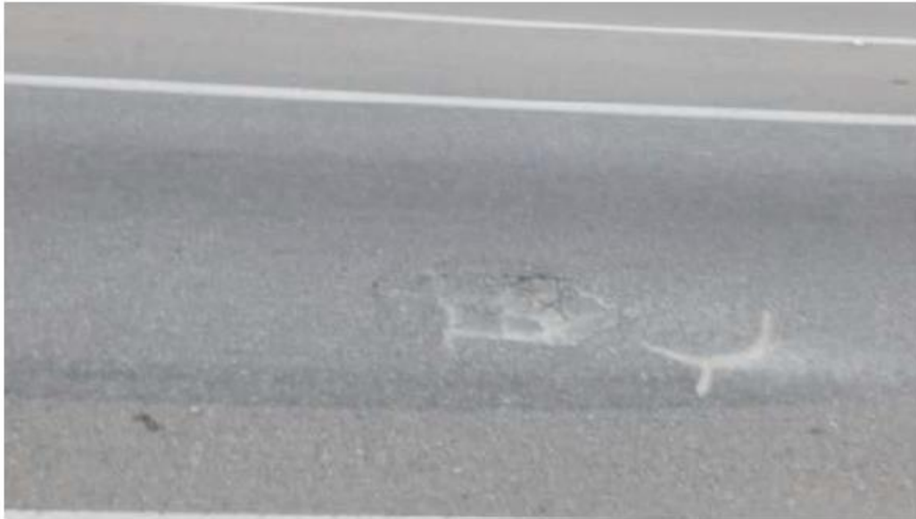
11 - Distressed area on asphalt pavement
