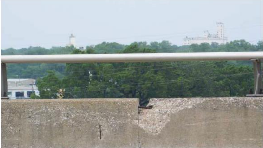
9 - Spall on East parapet
