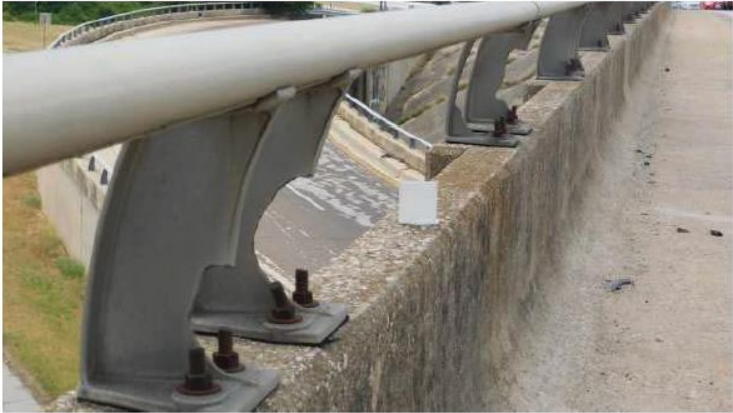
10 - Broken rail posts on West bridge rail
