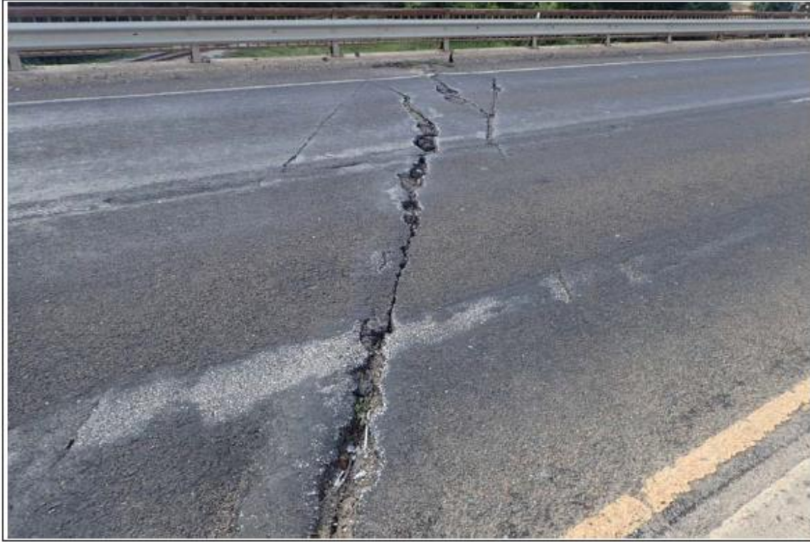
Photo 15 - Asphalt over Bent 7, full width x up to 9" L x 3" D transverse crack with spalling, looking east
