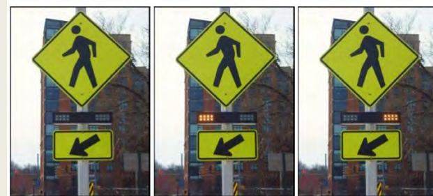
Figure 1. Example of an RRFB dark (left) and illuminated during the flash period (center and right) mounted with W11-2 sign and W16-7P plaque at an uncontrolled marked crosswalk.
