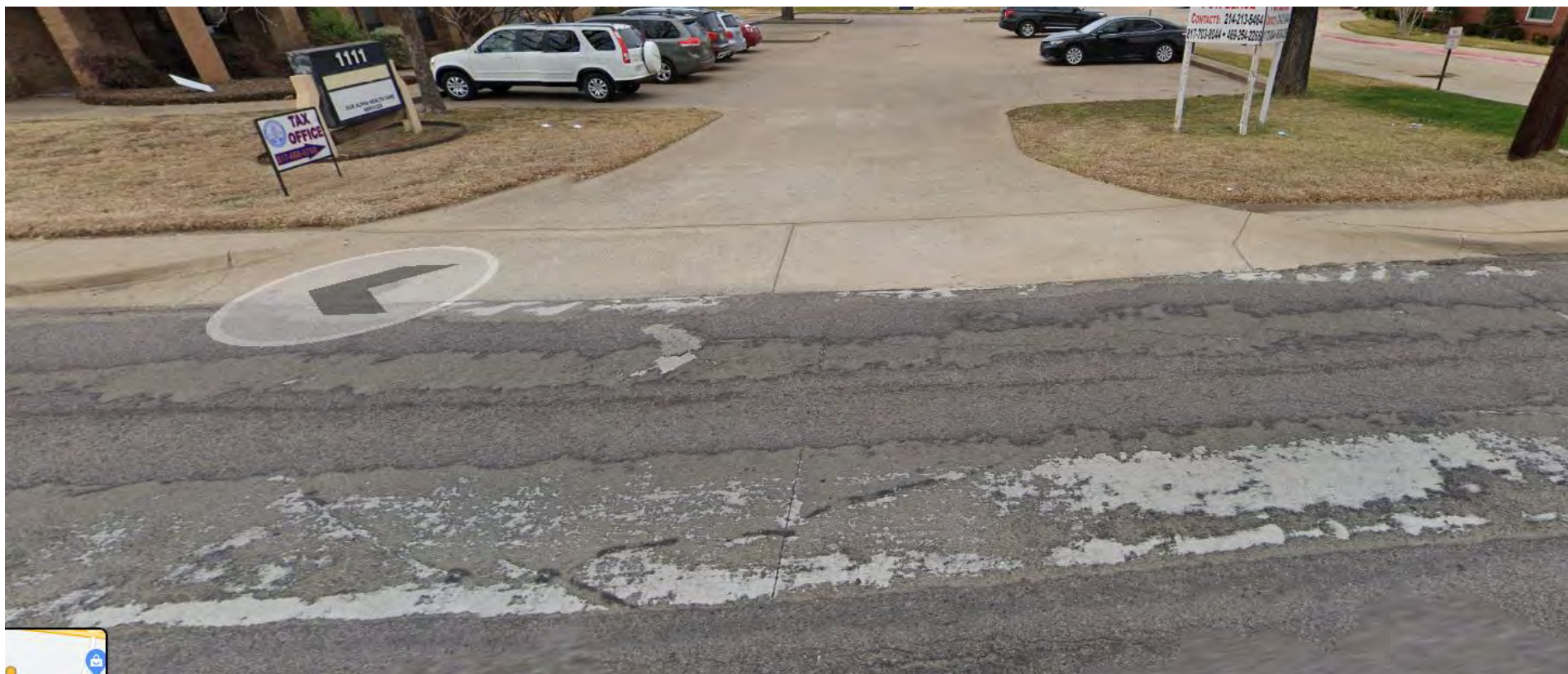
Figure 4: (Westbound along W Arkansas Ln) - Access points along the route with no ADA compliance, narrow sidewalks, poor pavement conditions, etc.
