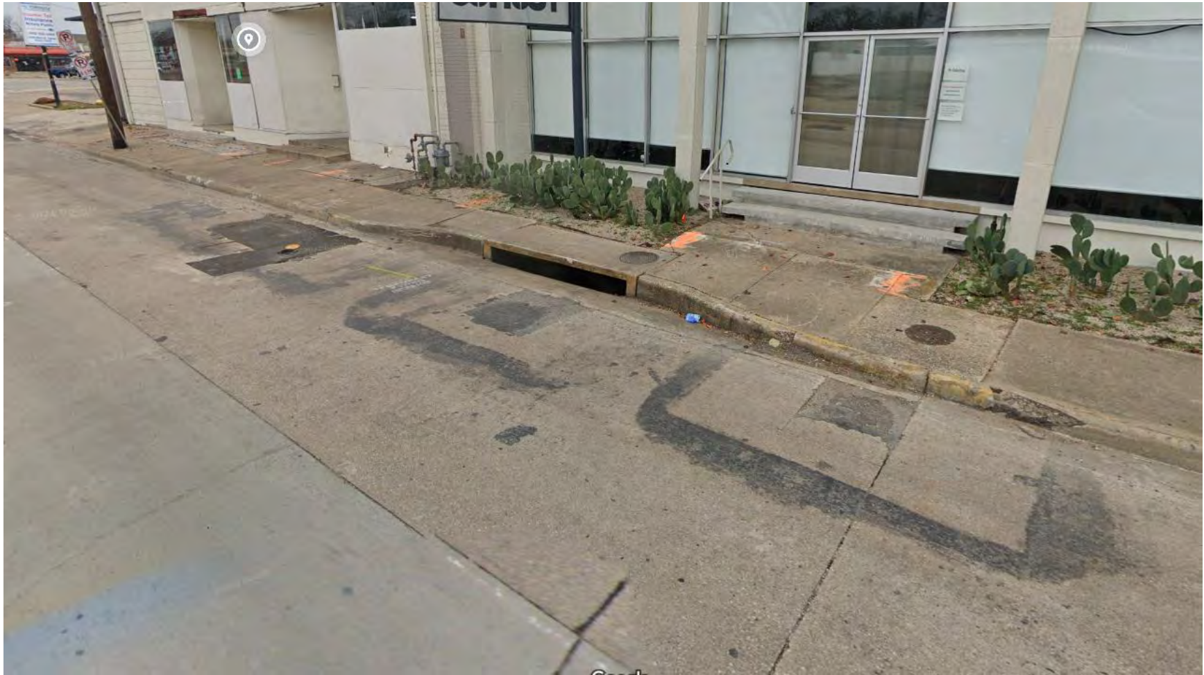
Figure 4: Narrow sidewalk sections and poor pavement conditions along segment.
