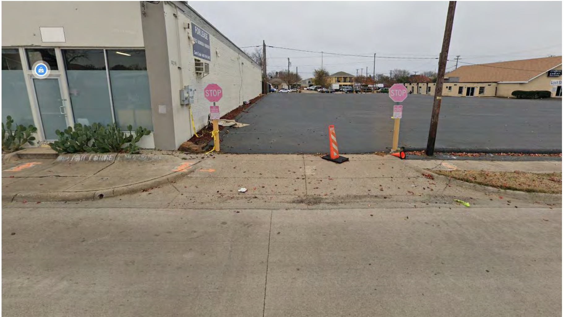
Figure 3: Driveways and access points with ADA compliance issues along segment.
