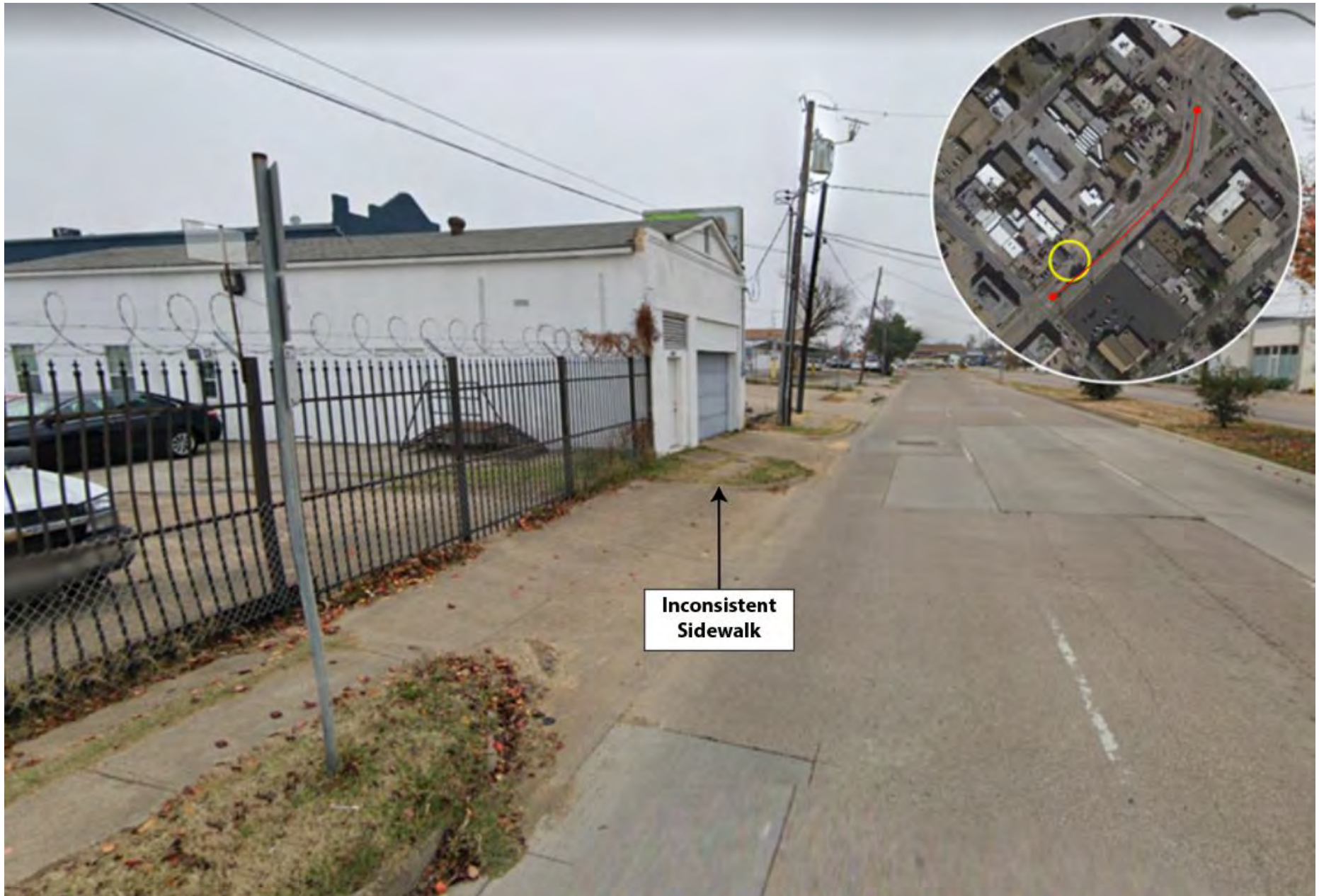
Figure 6: Pedestrian facilities near the intersection of Main and Peak: Sections of sidewalk lacking ADA compliance, that periodically disconnect and force pedestrians to walk closer to the road and oncoming traffic. Utilities and abutting properties possess part of the existing sidewalk.
