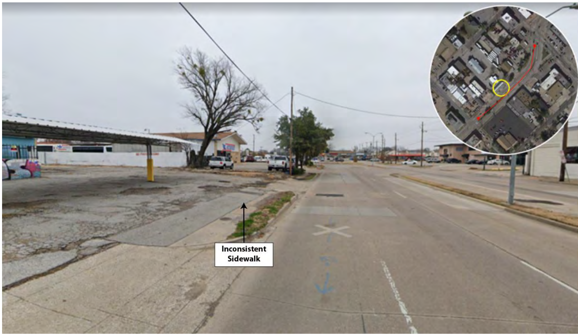
Figure 3: Pedestrian facilities halfway between Peak St and Carroll St have inconsistent and disconnected sidewalks that lack ADA compliance. Sidewalk and abutting property need repaving, ROW planting needs maintenance, and utilities encroach on sidewalk.
