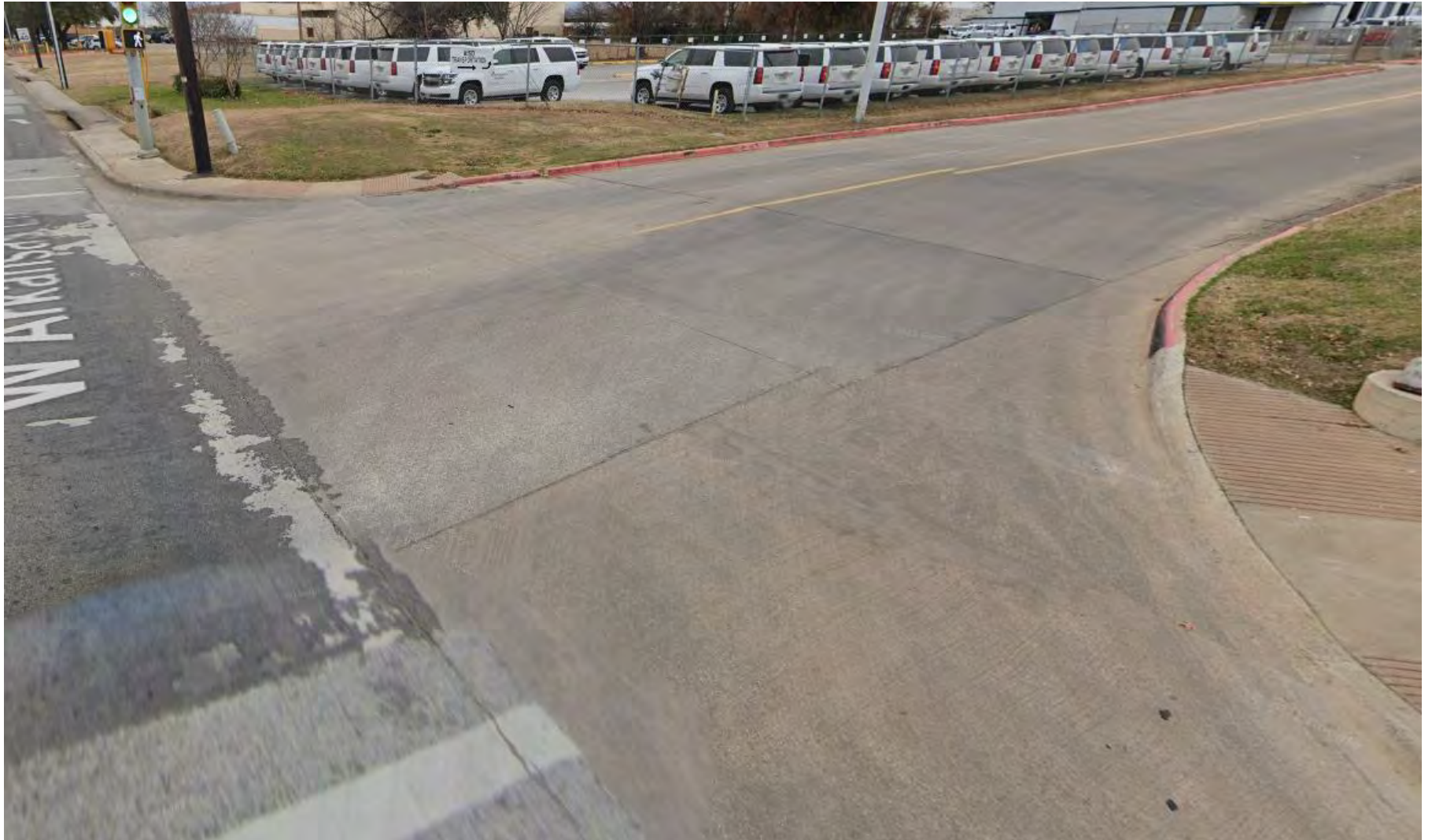
Figure 2: More pedestrian facilities at intersection of S Davis and Arkansas Ln: some sections lacking ADA compliance, no connected sidewalk facilities to Davis, utilities need to be relocated, narrow existing sidewalks, poor conditions, deficient crosswalk striping, etc.
