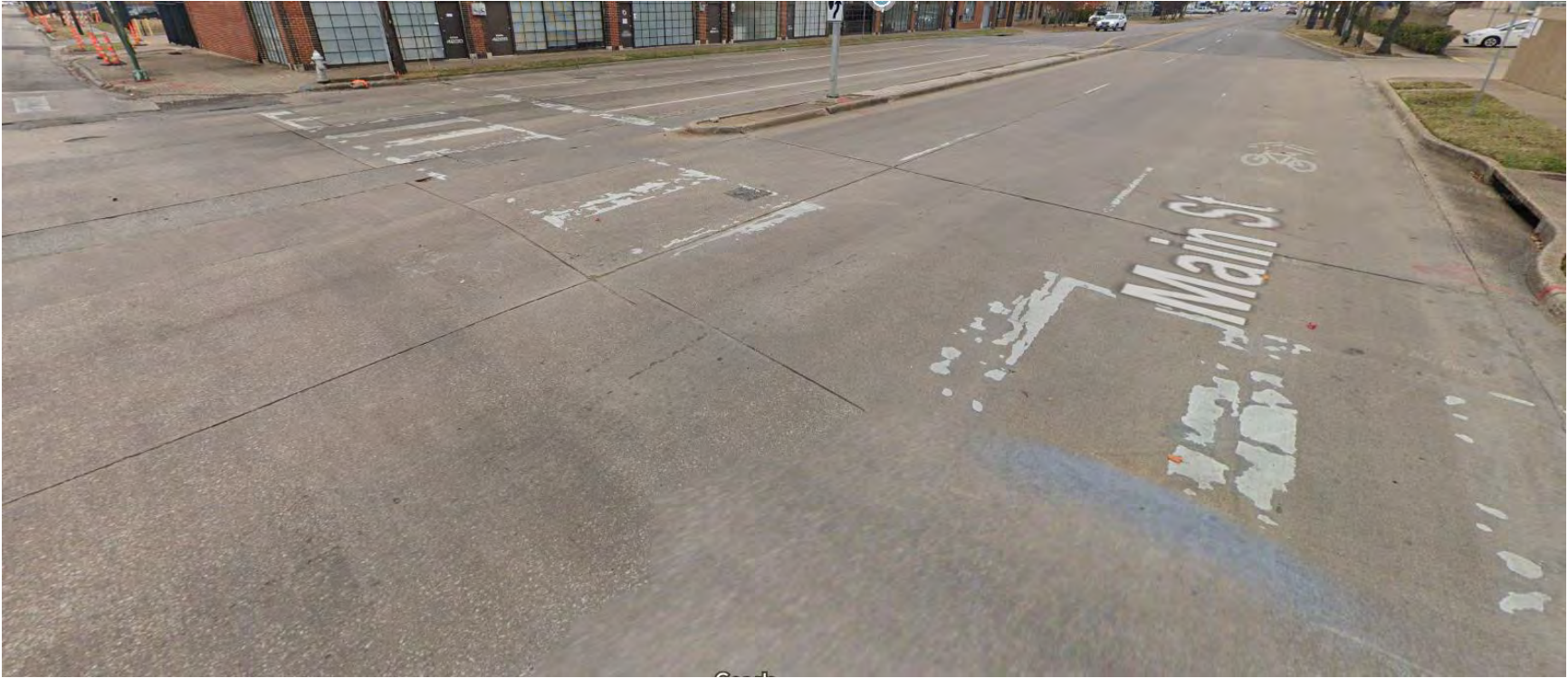
Figure 2: Intersection at Main St and Peak. Poor sidewalk conditions, cross walk striping, ADA compliance issues, utilities need to be moved, limited right-of-way, etc.
