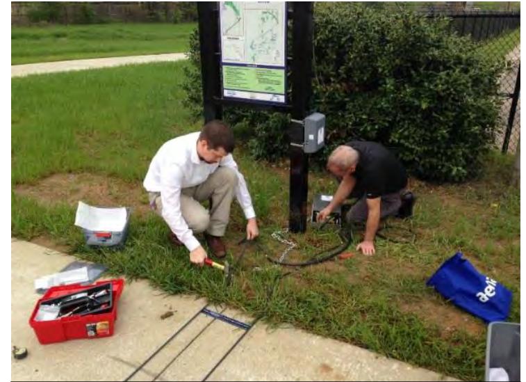
Installation of a mobile counter on the John Barfield Trail in North Richlands Hills
