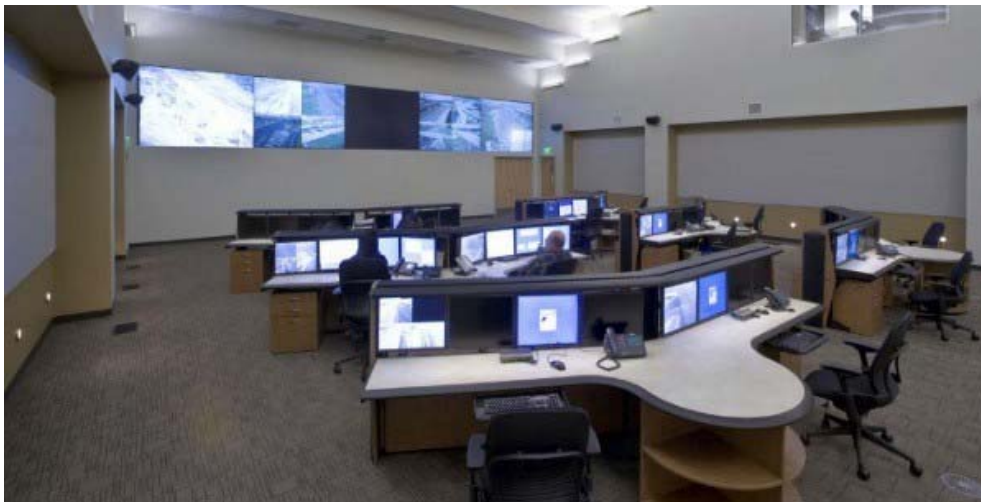
TxDOT Dallas District TMC
