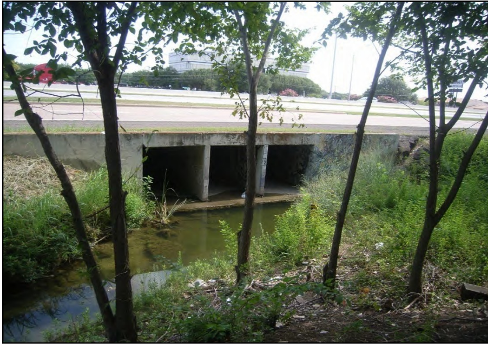
Photograph 17: Representative photograph of stream flowing to culvert along US 80. View is to the east-northeast. (8/10/2017)
