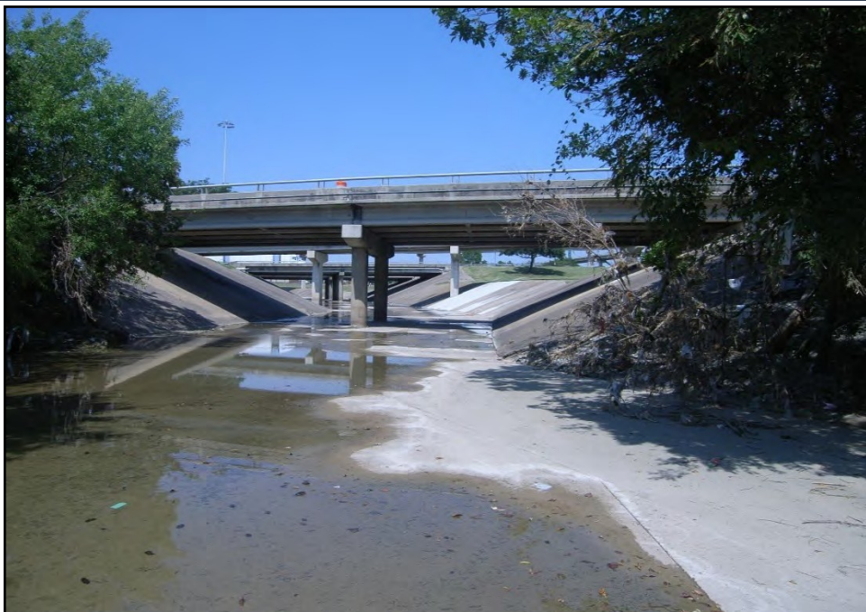
Photograph 18: Representative photograph of a concrete lined channel flowing under bridged section of US 80. View is to the north-northeast. (9/14/2017)
