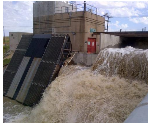
Pavajo Pump Station on Canada Drive
