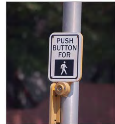
FIGURE 58: PEDESTRIAN SIGNAL DEVICE
