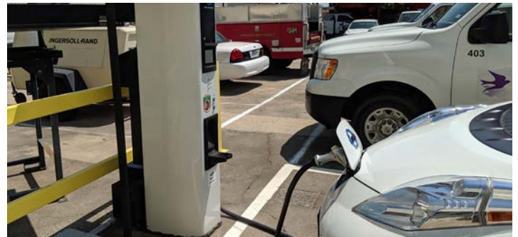
City of Lewisville's DCFC Charging Station on Their Fleet Lot.
