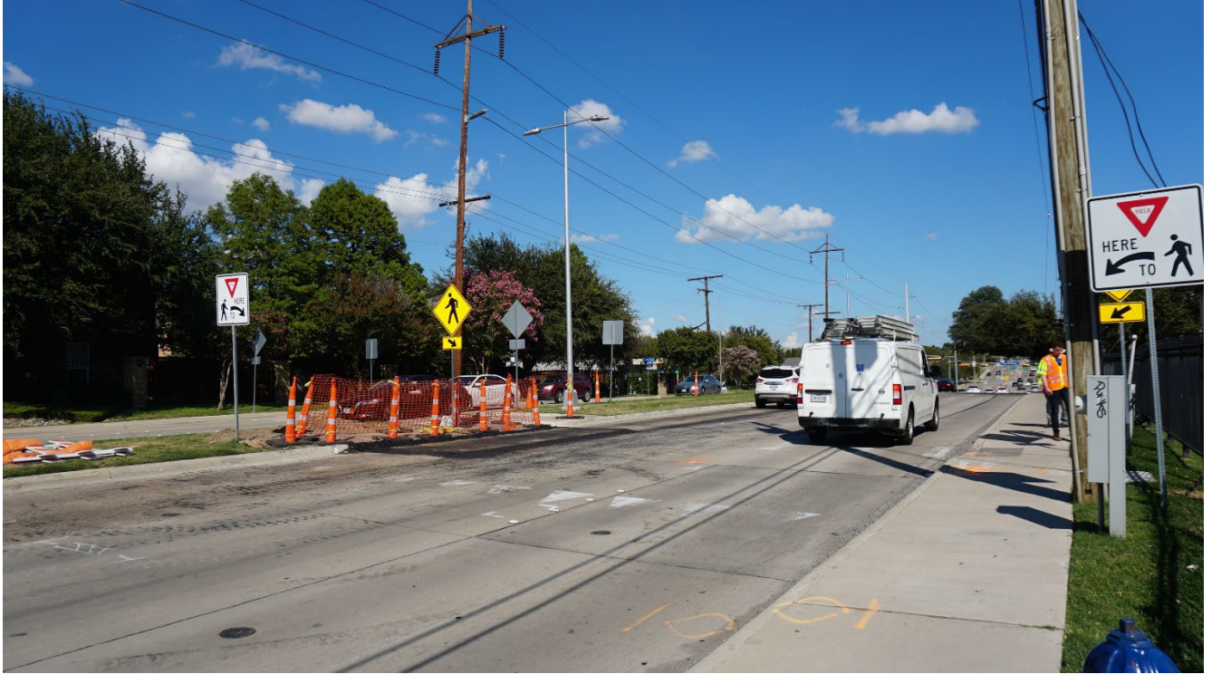
Figure 9: Closure of midblock crossing with no warning or accessible detour path
