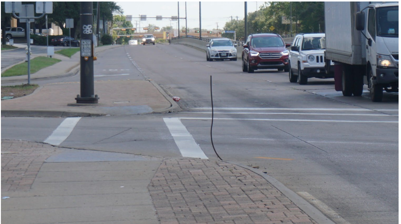
Figure 23: Rebar obstruction on sidewalk/curb
