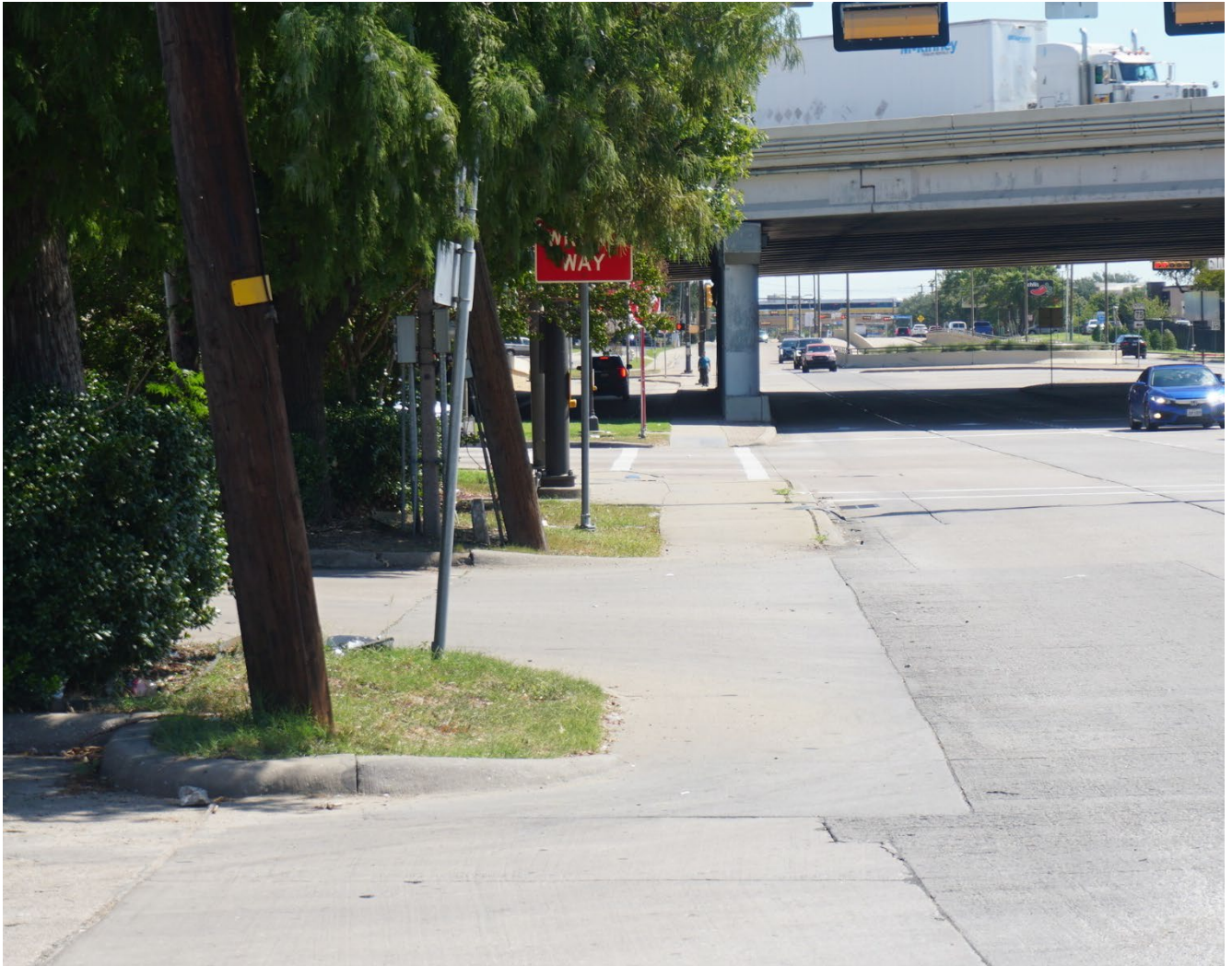
Figure 28: Missing or ambiguous sidewalk
