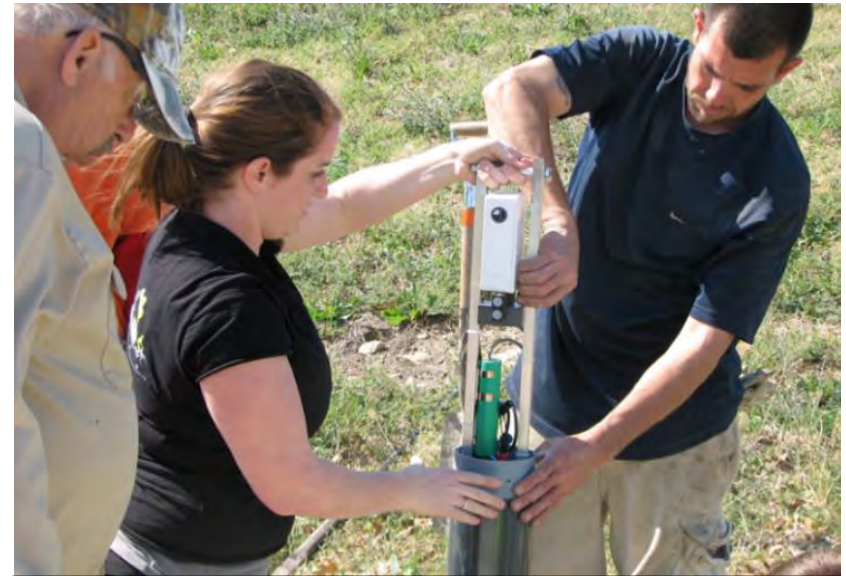
Installation of a permanent count station in Fort Worth.
