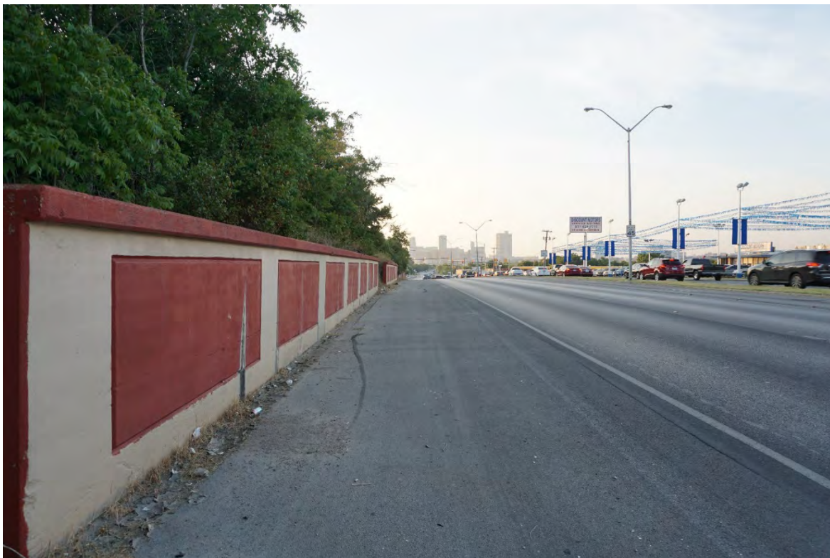
Figure 4. Photograph of SH 199 Looking East Along Concrete Retaining Wall Source: Freese and Nichols, Inc., 2016
