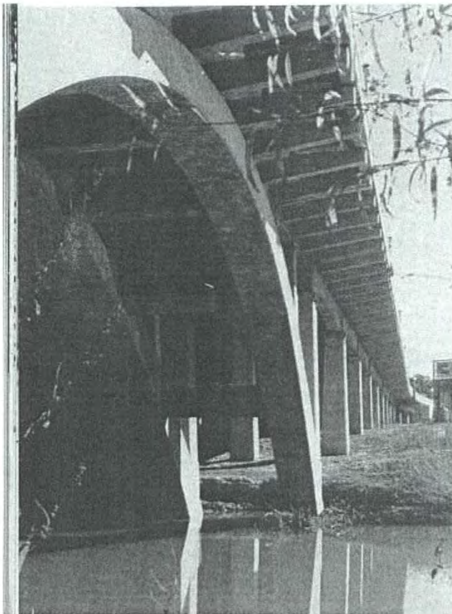
Figure 4: photo of Henderson Street Bridge from the August 1937 edition of Fort Worth's Municipal Life .
