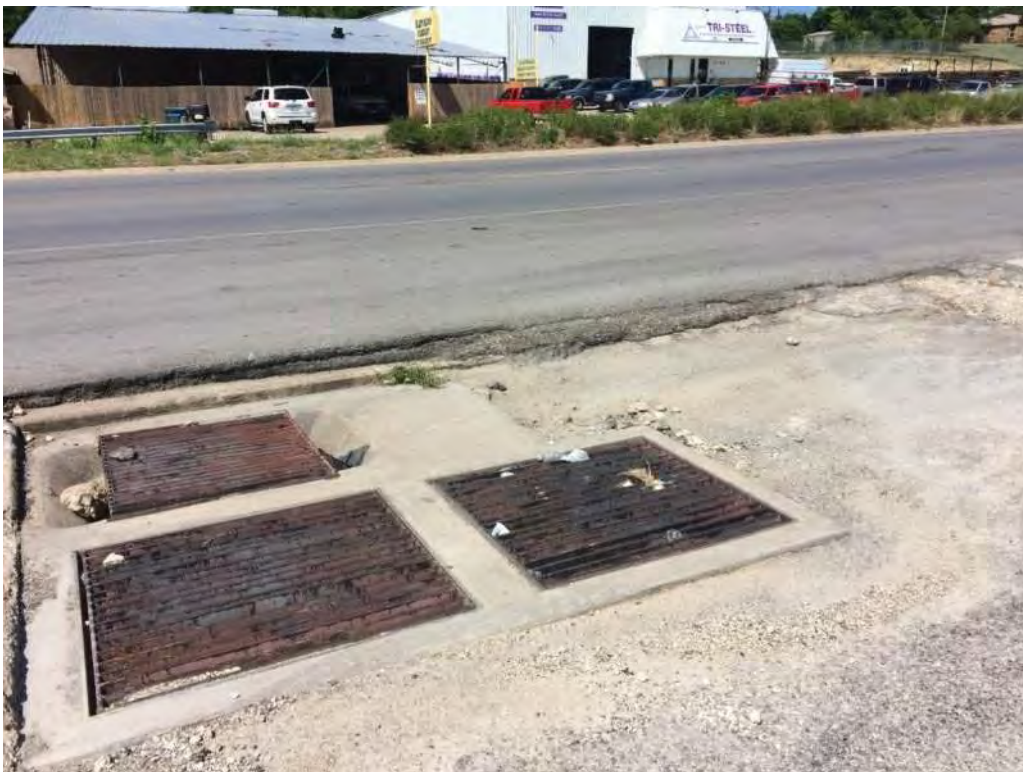
Inlets at Jacksboro Highway Sansom Park; No Curb and Gutter
