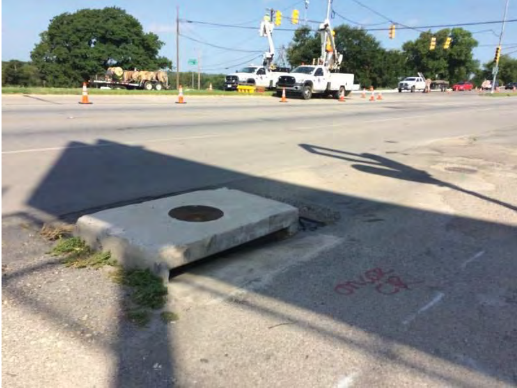
Inlet at Jacksboro Highway in Fort Worth near Grand Avenue; No Curb and Gutter
