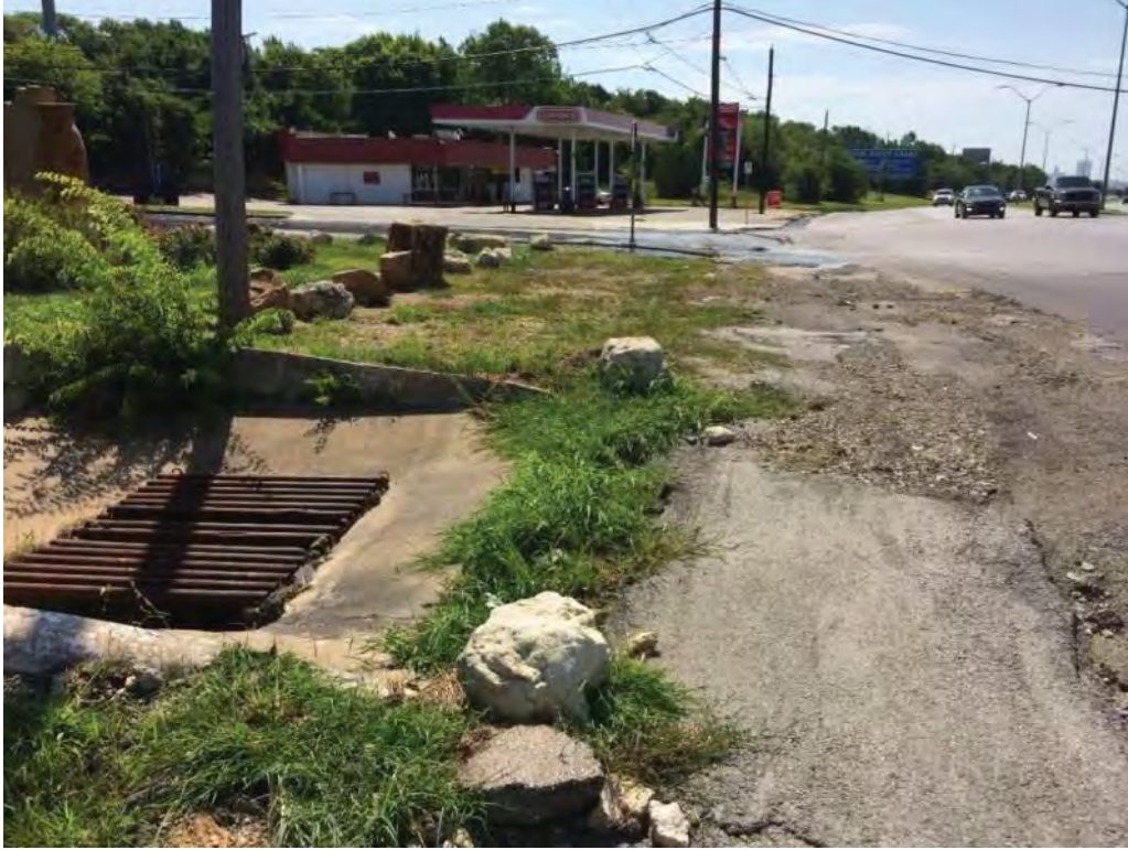
Inlet at Jacksboro Highway Near Beverly Hills Drive in Sansom Park; No Curb and Gutter
