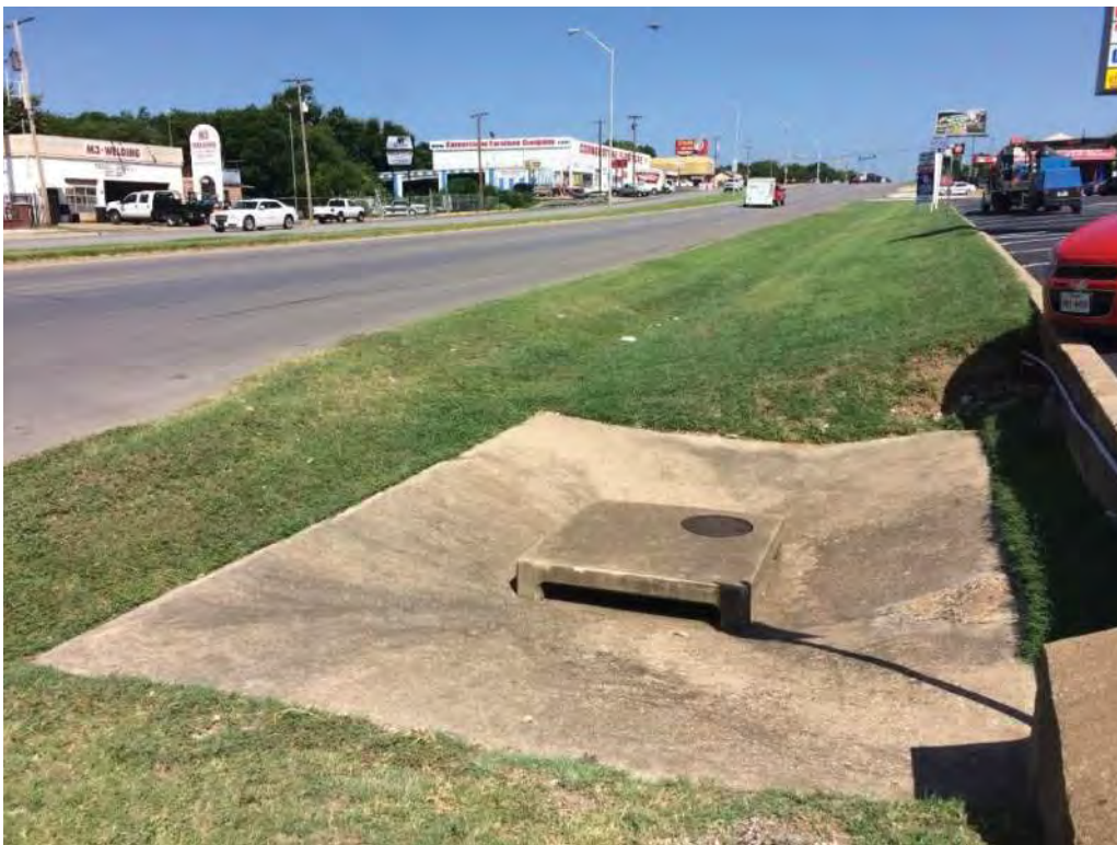
Inlet and Ditch at Jacksboro Highway in Fort Worth; No Curb and Gutter
