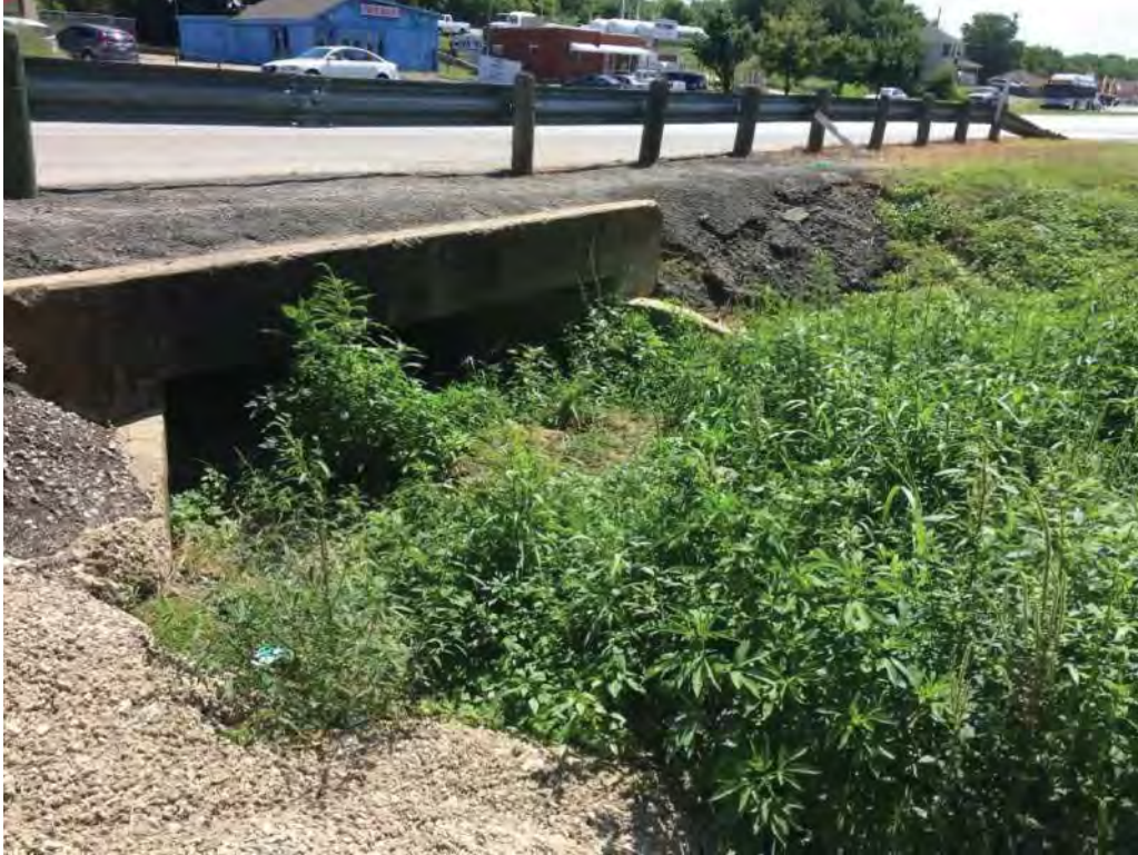
Silted Culvert at Jacksboro Highway in Sansom Park; No Curb and Gutter
