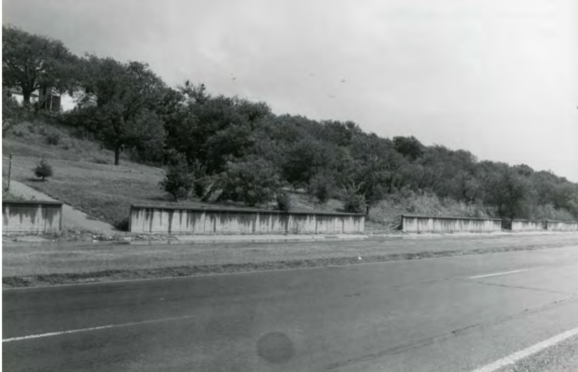
Figure 3. Photograph of SH 199 Looking North at Concrete Retaining Wall Source: National Register of Historic Places, 1987
