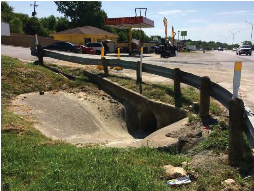
Culvert and Ditch at Jacksboro Highway Near Skyline Drive in Sansom Park; No Curb and Gutter
