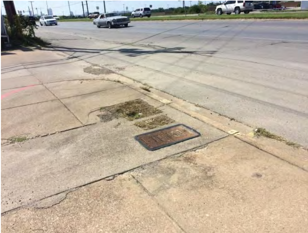
Jacksboro Highway with Curb and Gutter in Fort Worth near Ephriham Avenue
