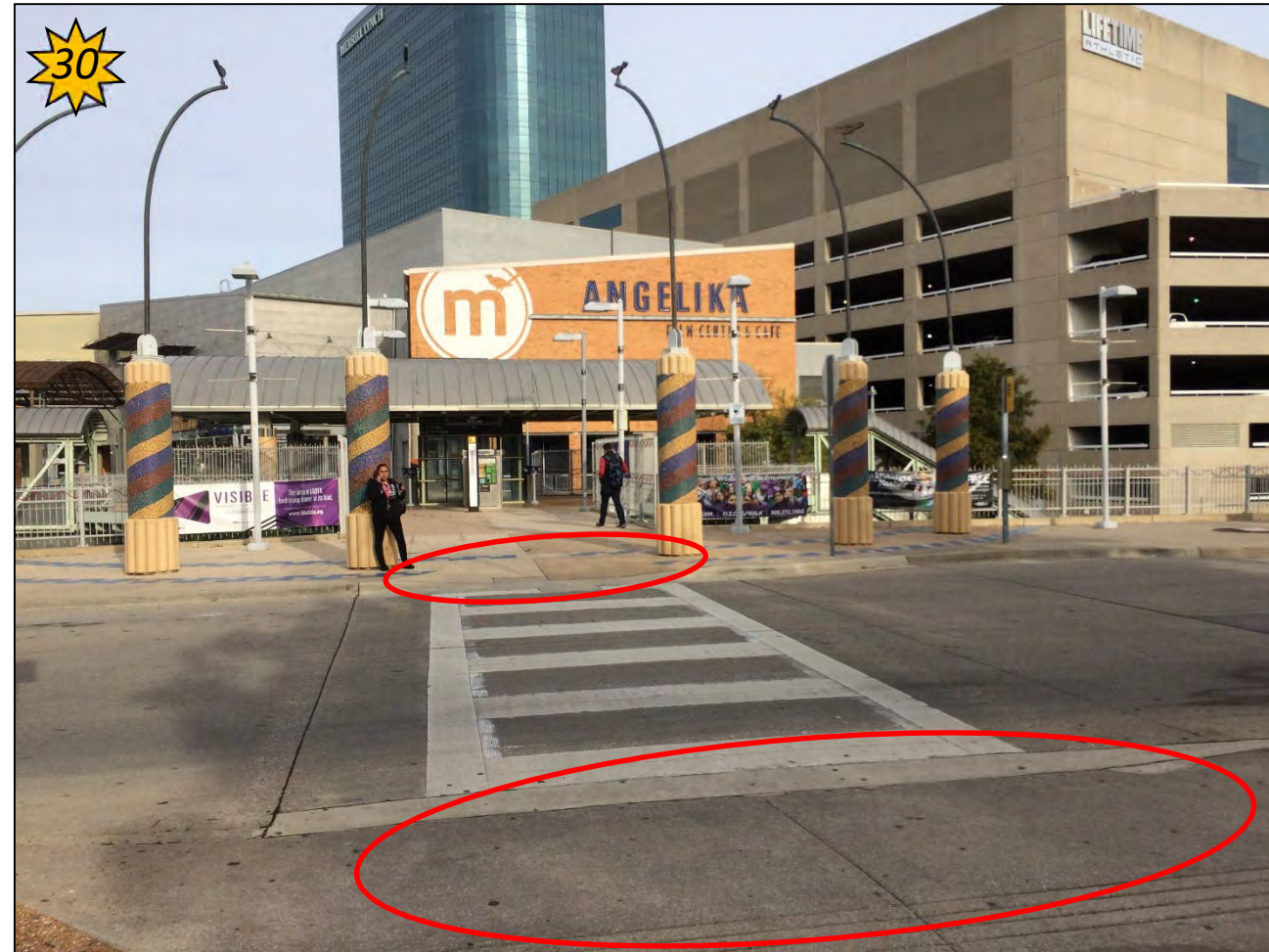
Add detectable warning surfaces to pedestrian ramps where missing. The above location is one example. Several others exist throughout the station area.
