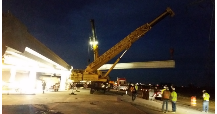
Beam setting on Thoroughfare B, the U-Turn Lane South of the Spring Creek Parkway.
