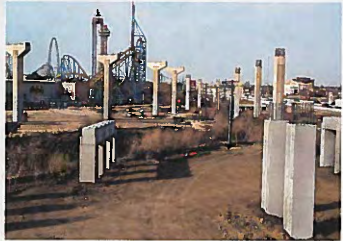
Bridge column construction on the I-30/SH 360 Interchange Project in Arlington. The $233 million project will increase safety, connectivity and mobility for motorists.
