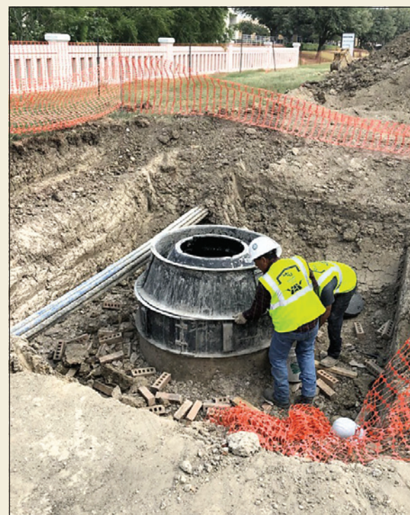
COURTESY OF THE CITY OF COPPELL Construction teams continue working on the South Belt Line reconstruction in preparation for DART’s Silver Line installation.
