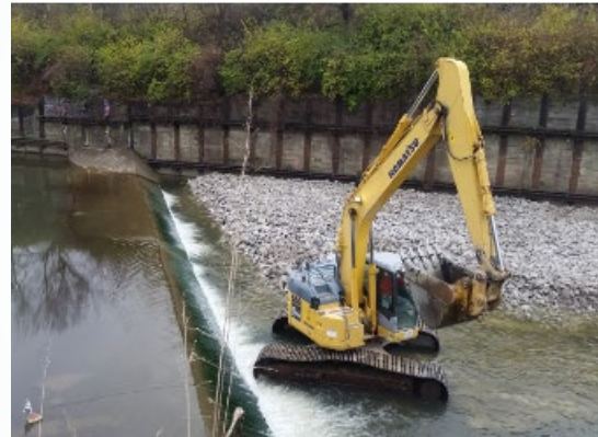
During: Addition of rock riffles downstream of the dam to raise the water level
