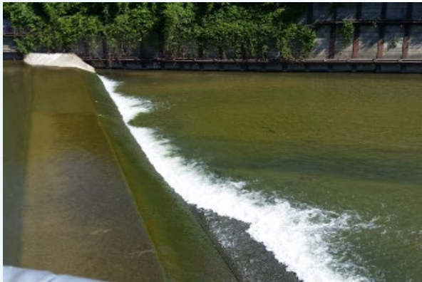
Before: Low-head dam near Cincinnati, OH
