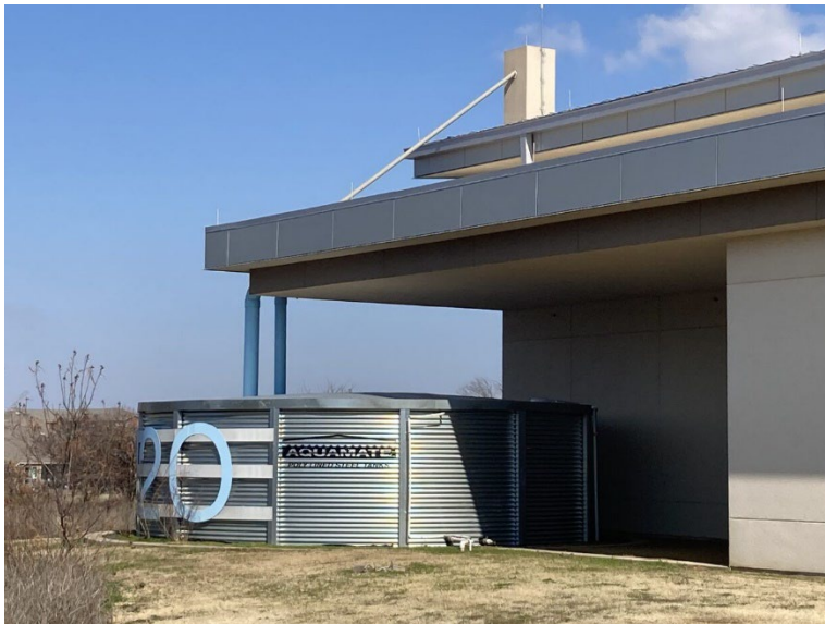
Figure 5. Rainwater harvesting system (Texas A&M AgriLife Extension Dallas Center, photo by Yufan Zhang)
