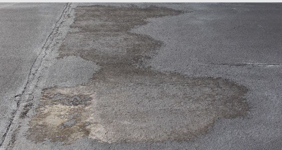
Oil Spillage (no severity)
