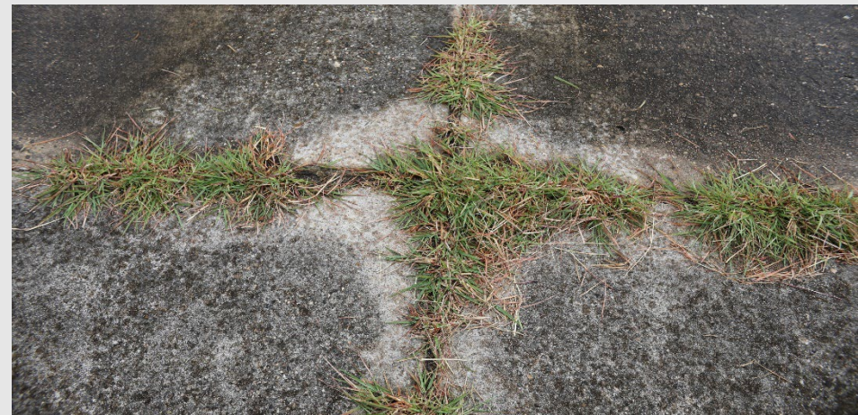
High Severity Joint Seal Damage
