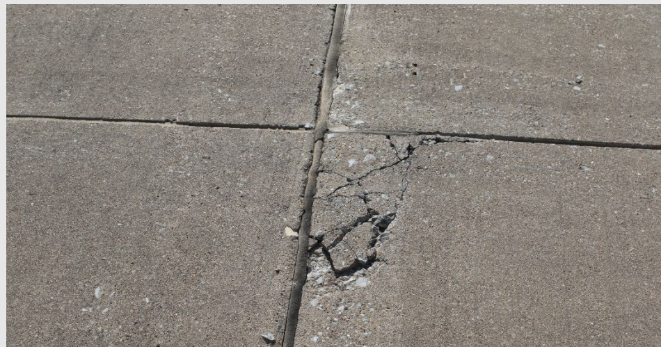
High Severity Corner Spall
