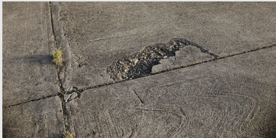
High Severity Joint Spall
