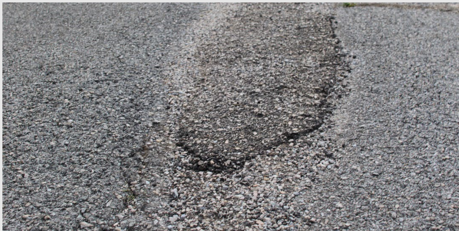
High Severity Patch
