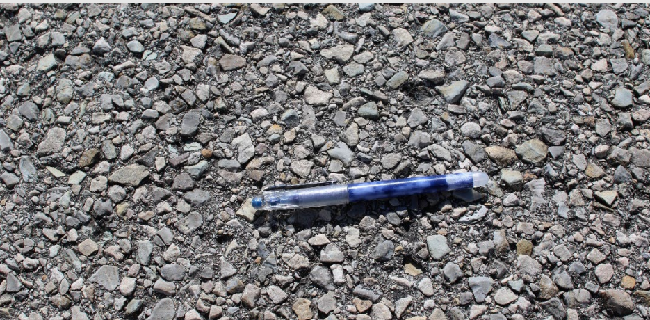
Medium Severity Weathering
