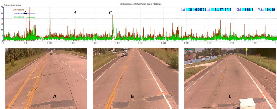
High Deflections in spall repair area
