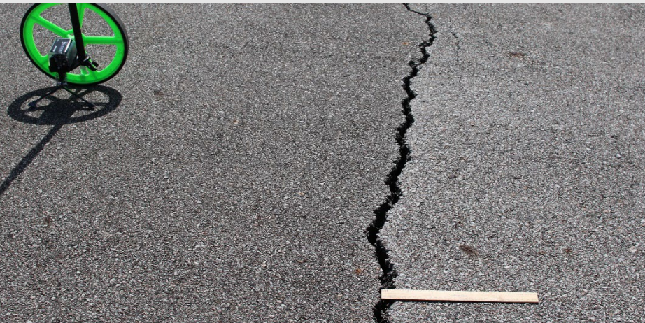
Medium Severity Longitudinal/Transverse Cracking
