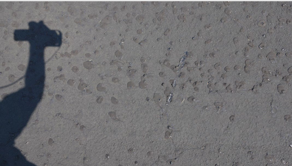
Bleeding (no severity)
