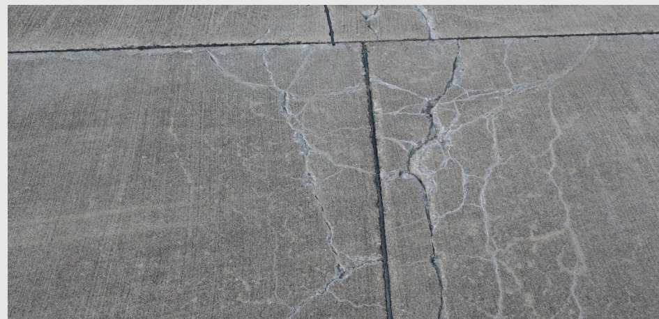
Medium Severity Durability Cracking
