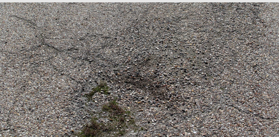
High Severity Raveling
