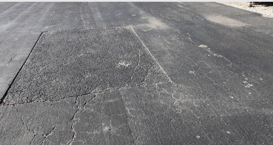
Medium Severity Patch
