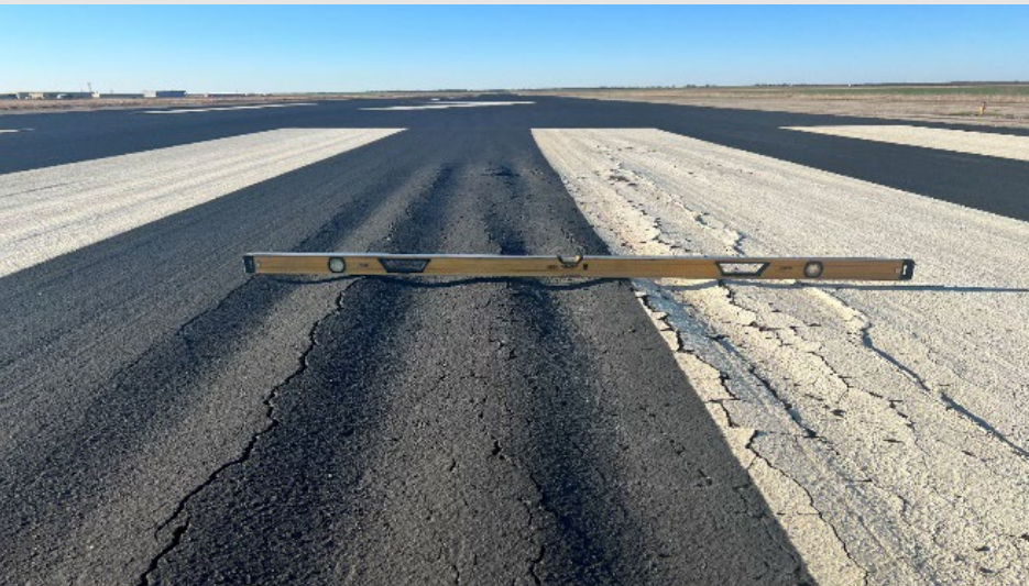
Medium Severity Rutting
