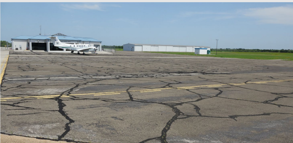
Low Severity Block Cracking
