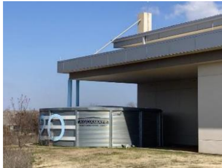
Rainwater harvesting (AgriLife)
