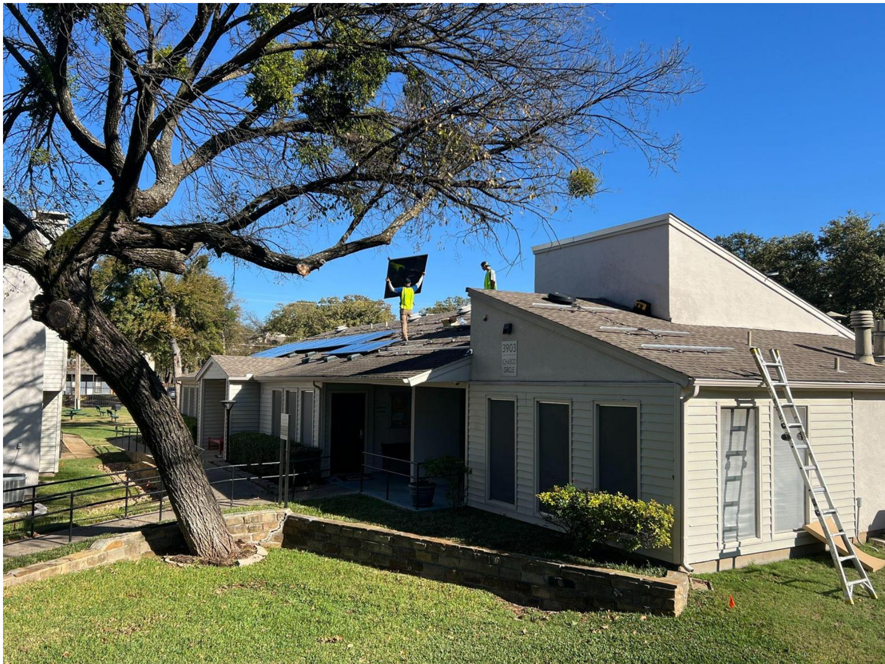
PV Installation, Family Solar- Sleepy Hollow Resilience Hub
