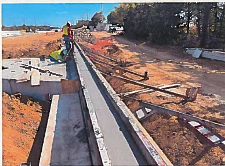
Crews work on the construction of a drainage structure on US 380 in Denton County
