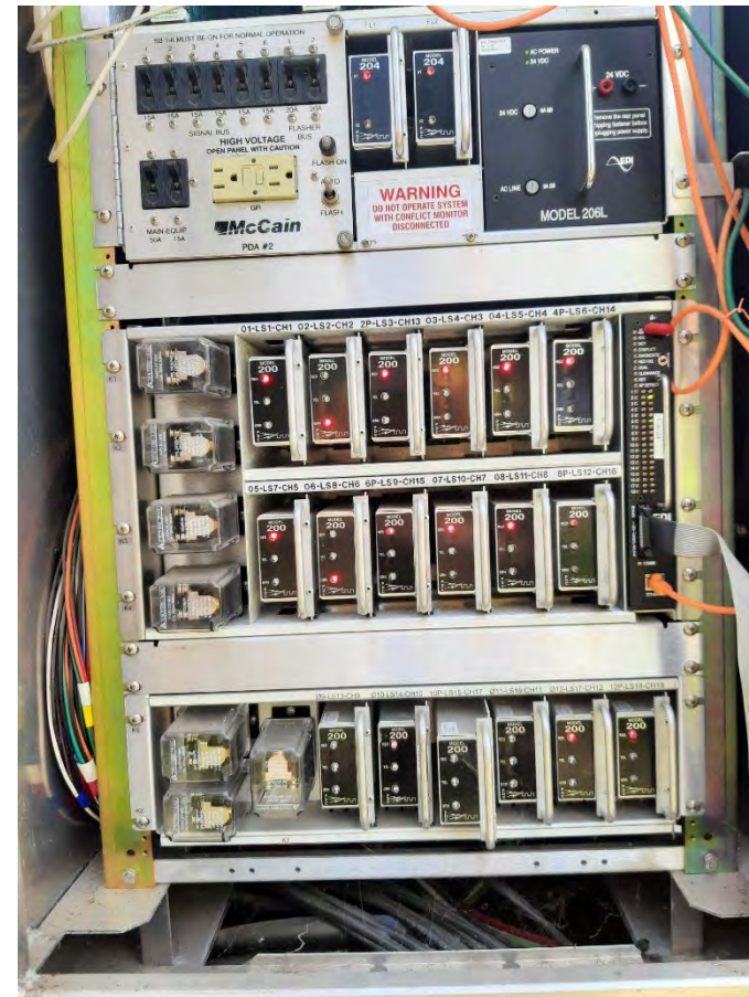
PHOTO OF CABINET LOAD SWITCHES
