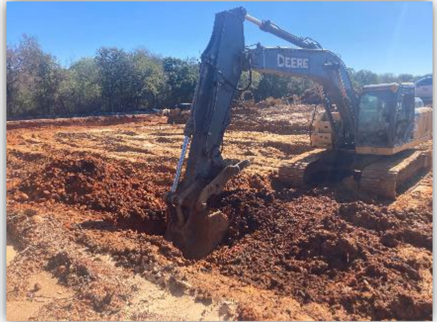
Test pit advanced along the northern border of the Site. View of the widespread excavation.
