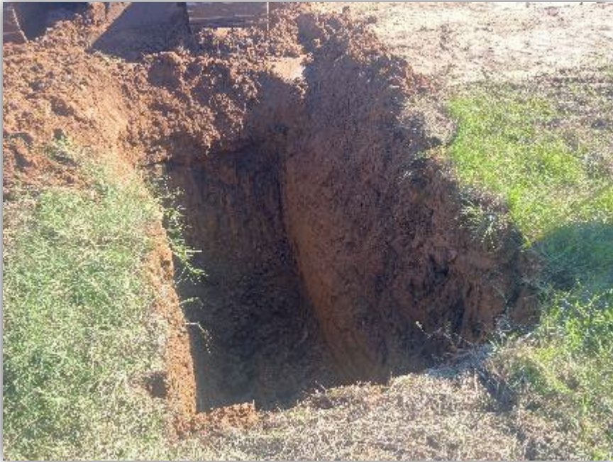
Test pit advanced in the mapped area of the NCTCOG landfill to eight feet bgs.
