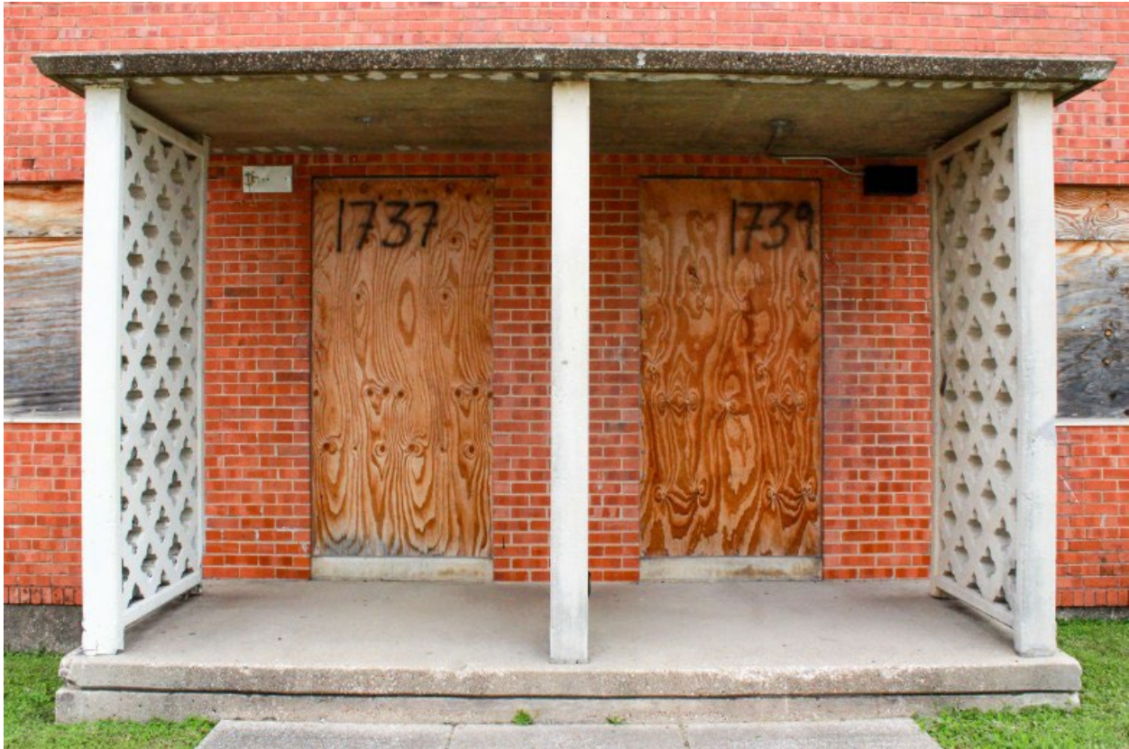
After the last tenants moved out in 2020, all doors and windows were boarded up. (Sandra Sadek | Fort Worth Report)
