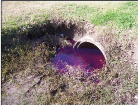
Field Investigation Example, Diesel spill - City of Grand Prairie (Photo courtesy of City of Grand Prairie, USA)
