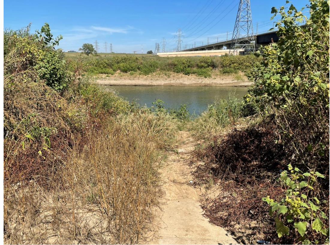
The ramp is in need of vegetation removal and silt removal
